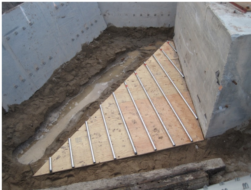
Figure 3-6: Photo of Concrete Wedge Roller System Under Wedges
