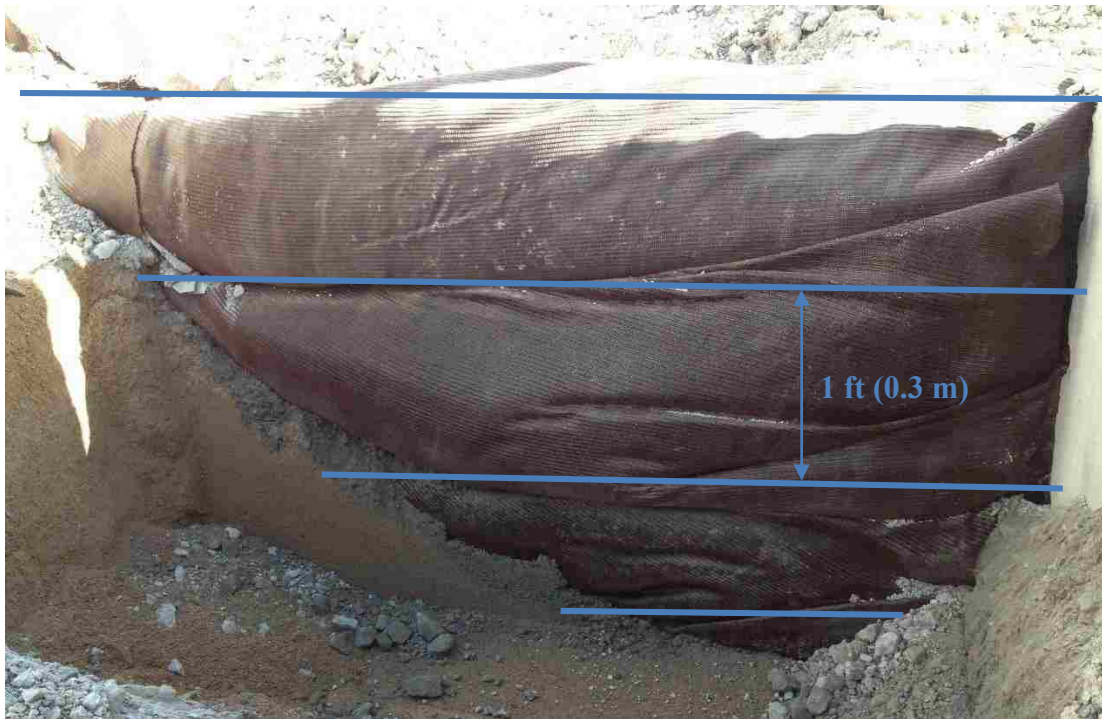
Figure 3-14. Geotextile fabric layer folds along the front of the backfill, made visible by removing the west transverse wingwall after testing.
