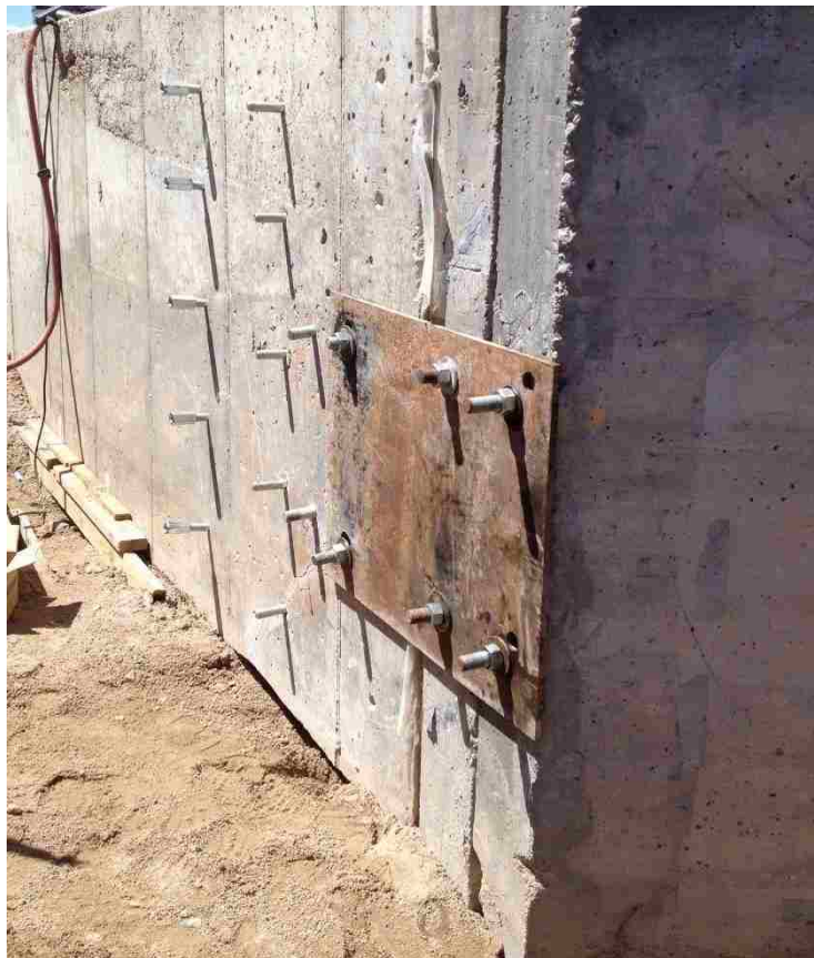
Figure 3-10. Example of metal plate and bolt connection for skew concrete wedges. The plate shown is located on the acute side of the pile cap.
