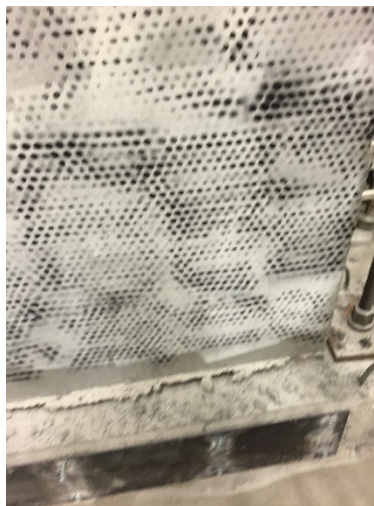
(b) Wall uplift.
