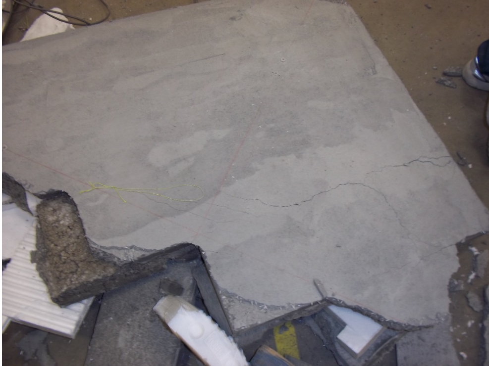
Figure 3-31 Wallette 8 after failure.
