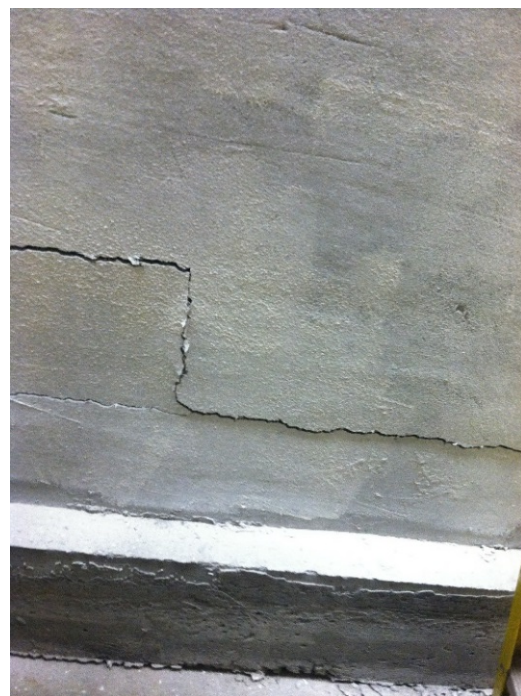
(b) Step down of horizontal crack to existing crack.
