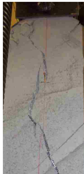
(b) Crack through face of wallette.
