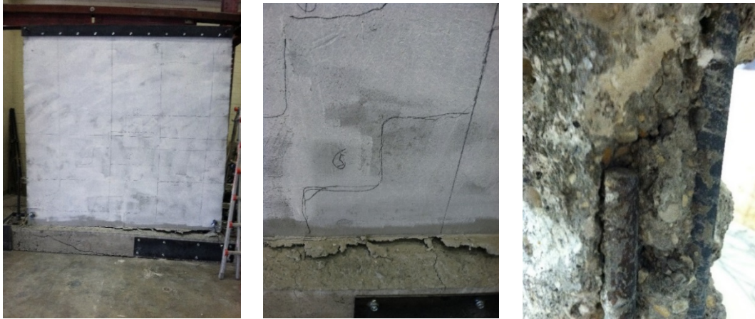
(a) Uplift of wall. (b) Typical diagonal cracks. (c) Pullout of dowel from grout.
