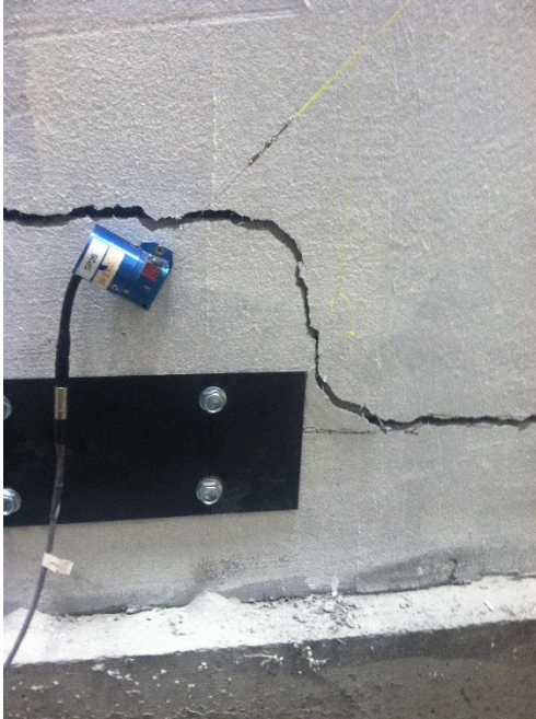
(a) Failure around steel plate.
