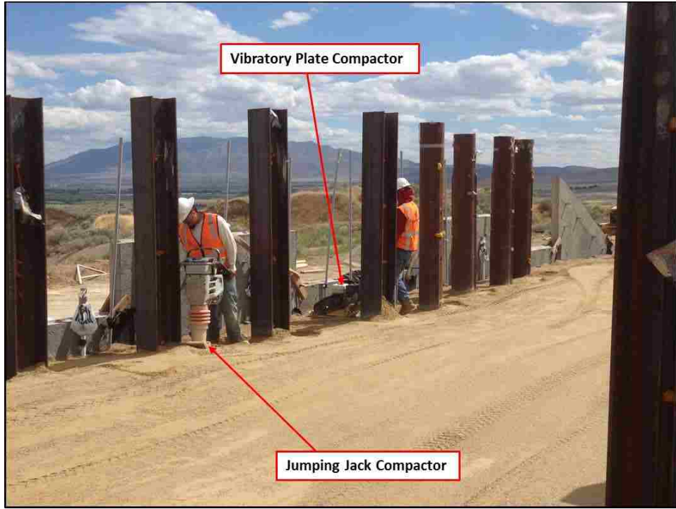
Figure 3-13: Compaction of backfill between the test piles and the back of wall using jumping jack and vibratory plate compactors.
