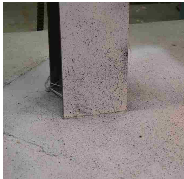
Figure 4-12: Yielded Column Flanges
