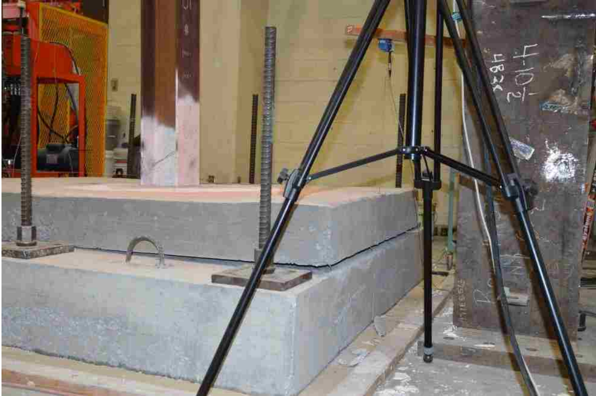
Figure 4-4: Slab Separation from Footing
