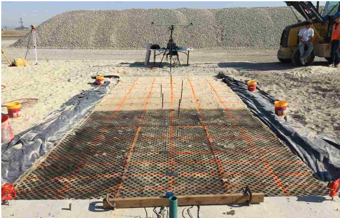
Figure 3-10: Uniform pattern of black dots painted on first 12 feet of backfill to aid the DIC camera system in tracking ground surface displacement
