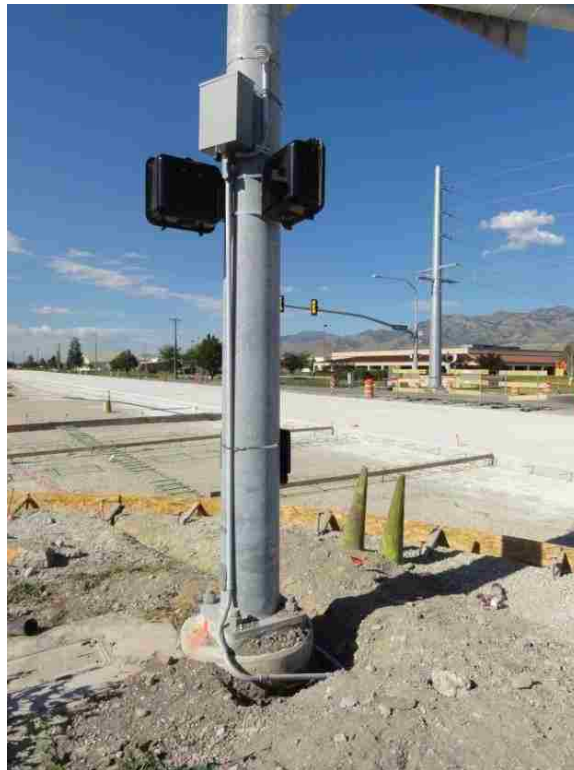
Figure 3-6: Utility box mounted on signal pole.
