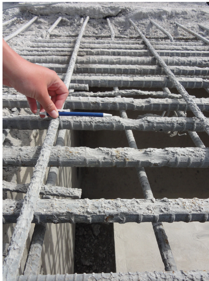
Figure 2-2: Corroded reinforcing steel in a concrete bridge deck.
