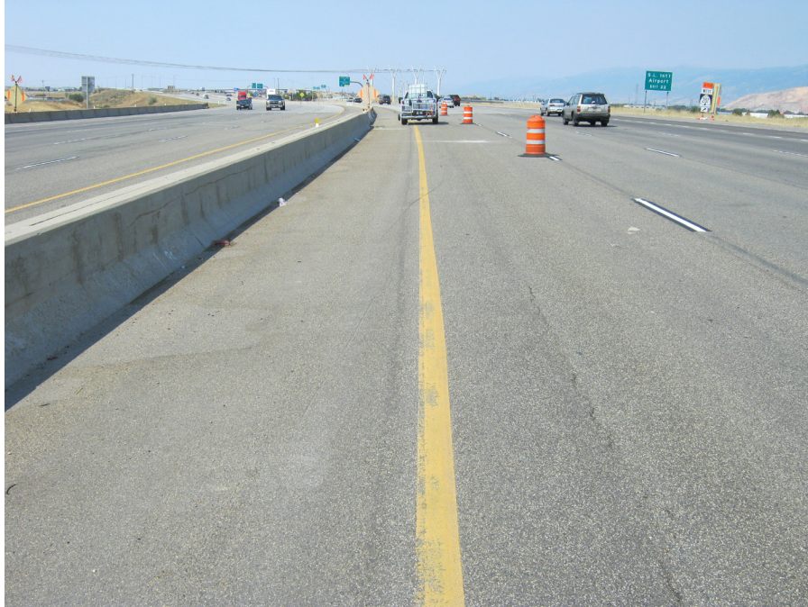
Figure 2-8: Cracking of asphalt overlay.
