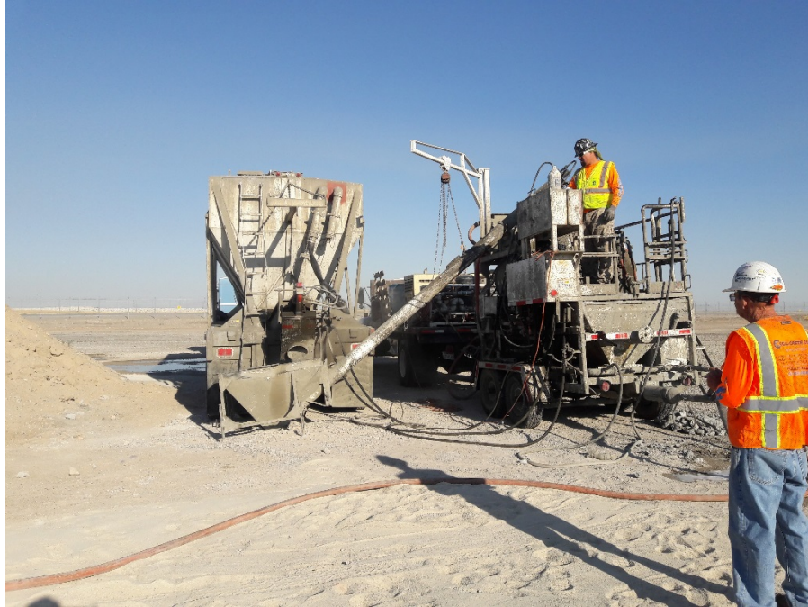
Figure 3-15: Production of cement slurry (truck on left) and the mixing with a specified amount of foam (unit on right) for the 0° skew backfill.
