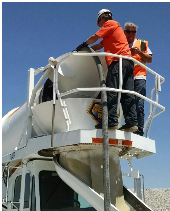
Figure 3-14: Addition of foam to cement slurry in cement truck for the 30° skew test backfill.
