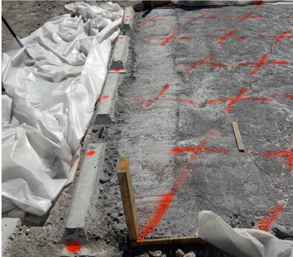
Figure 3-8: Flowable fill (CLSM) placed between backfill and reaction block wall to alter test site layout.
