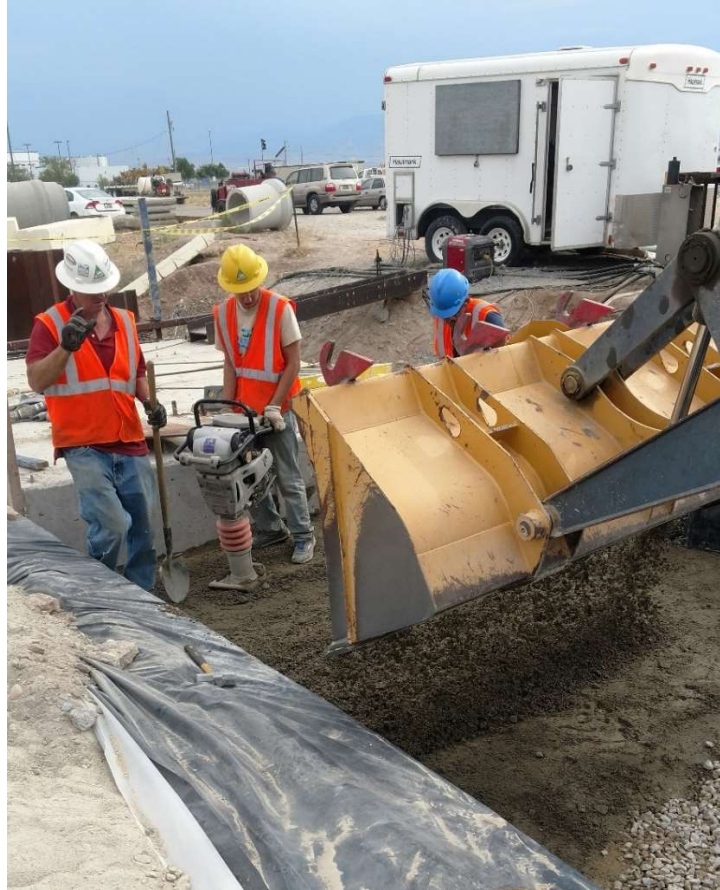
Figure 3-9. Backfill was dumped by backhoe into box, then spread by shovel before compaction.
