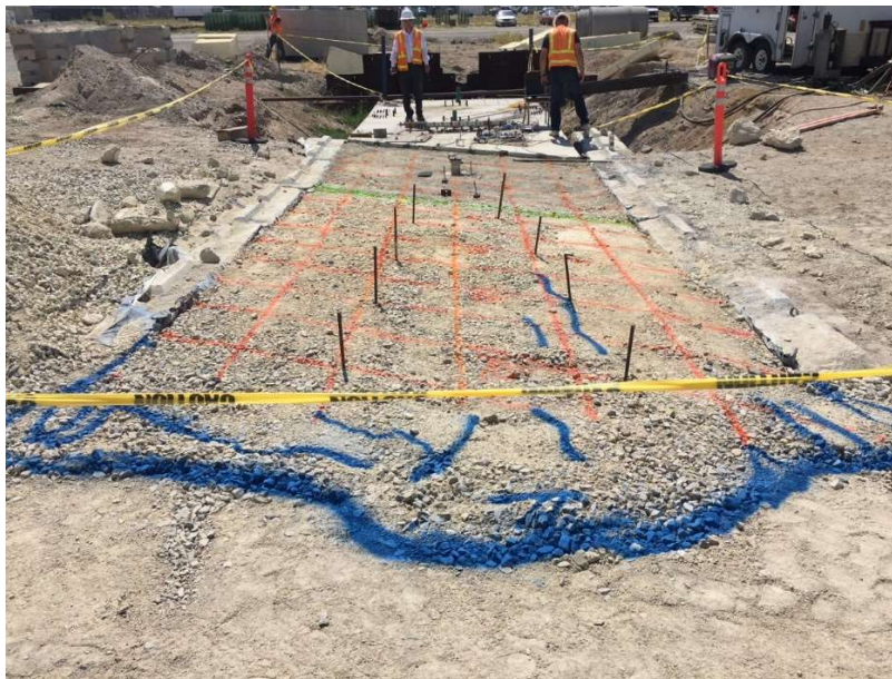
Figure 3-31. 30° skew after passive loading test, showing grid lines in orange and surface cracking highlighted in blue.
