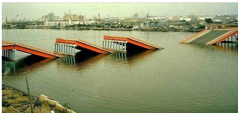
Figure 4-1: Example of lateral spread displacements causing bridge spans of the Showa Bridge in Niigata, Japan, to lose support and collapse in after the 1964 earthquake (after Bhattacharya et al. (2014)).
