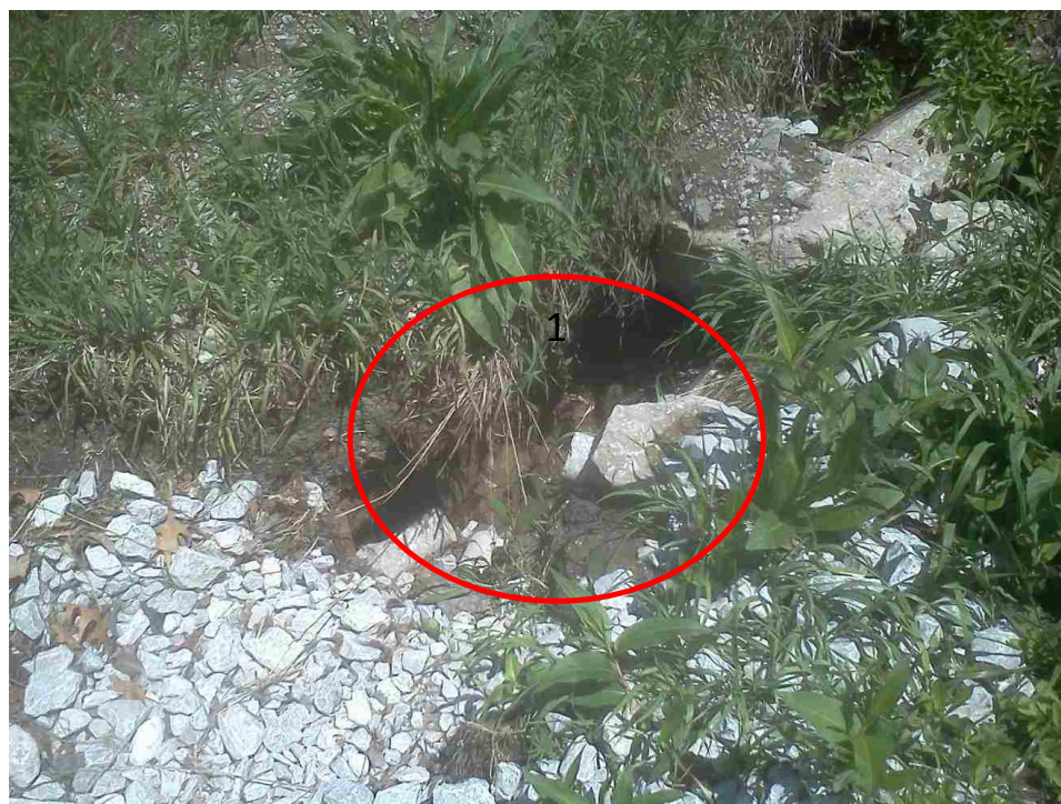
Figure 2.23 Filter trench undermining at beginning of trench
