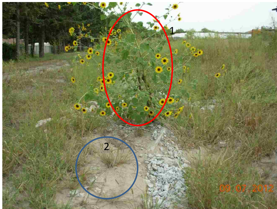
Figure 2.22 Filter trench sediment buildup and vegetative growth
