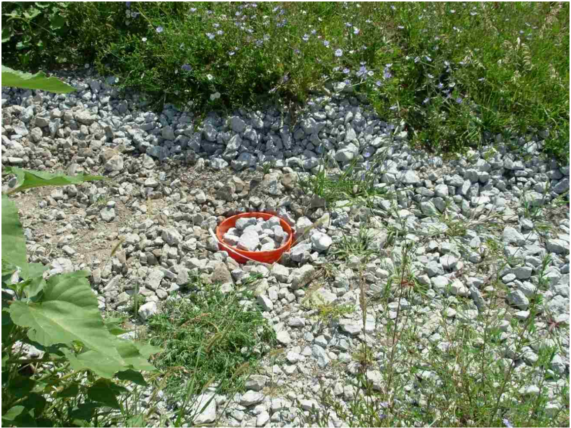
Figure B.12 Sediment bucket in infiltration trench
