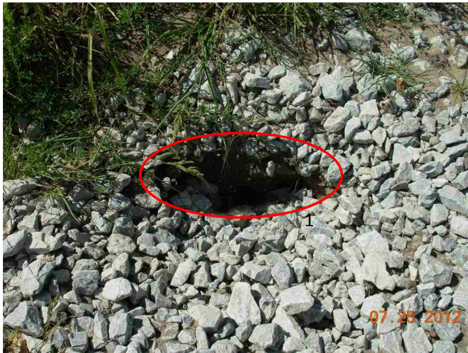
Figure 2.25 Filter trench undermining hole along trench
