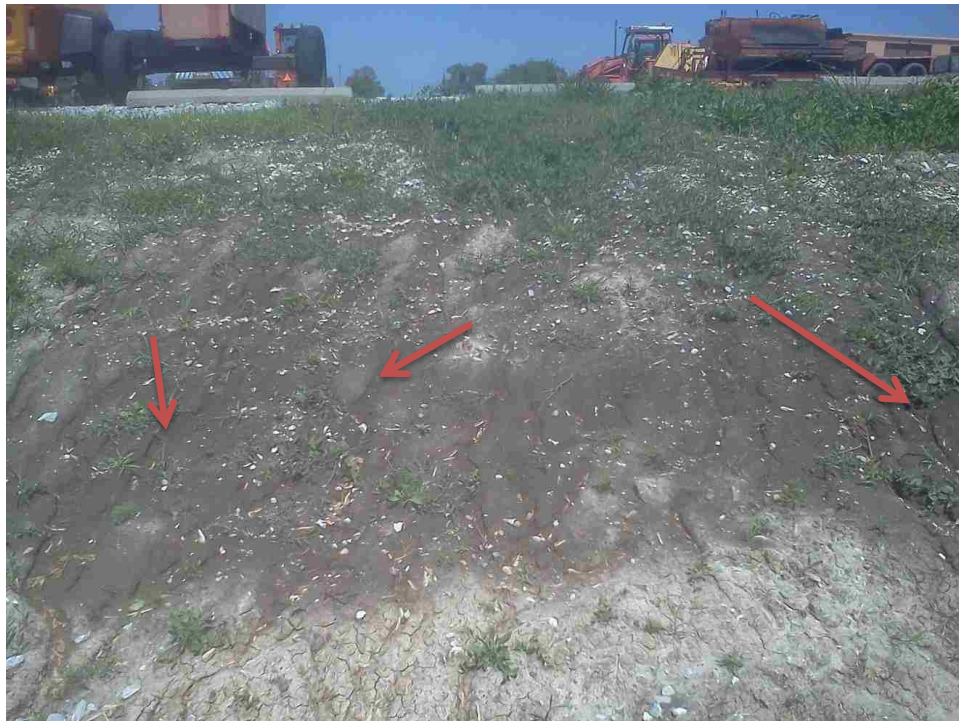
Figure 2.20 Filter trench side slope rills
