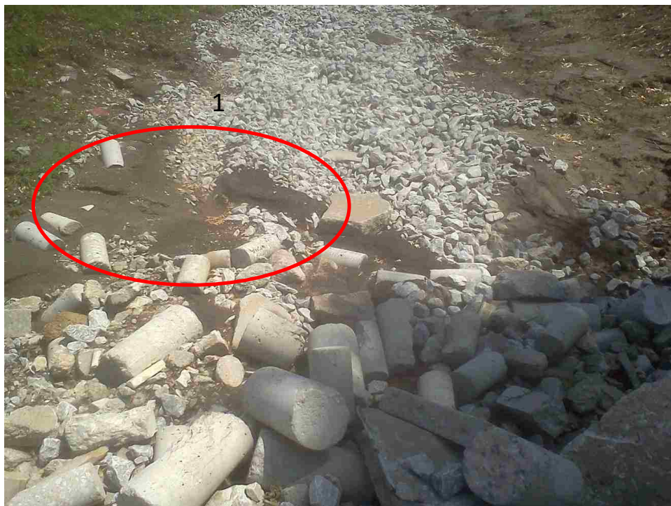
Figure 2.21 Filter trench sediment buildup on armoring and check dams
