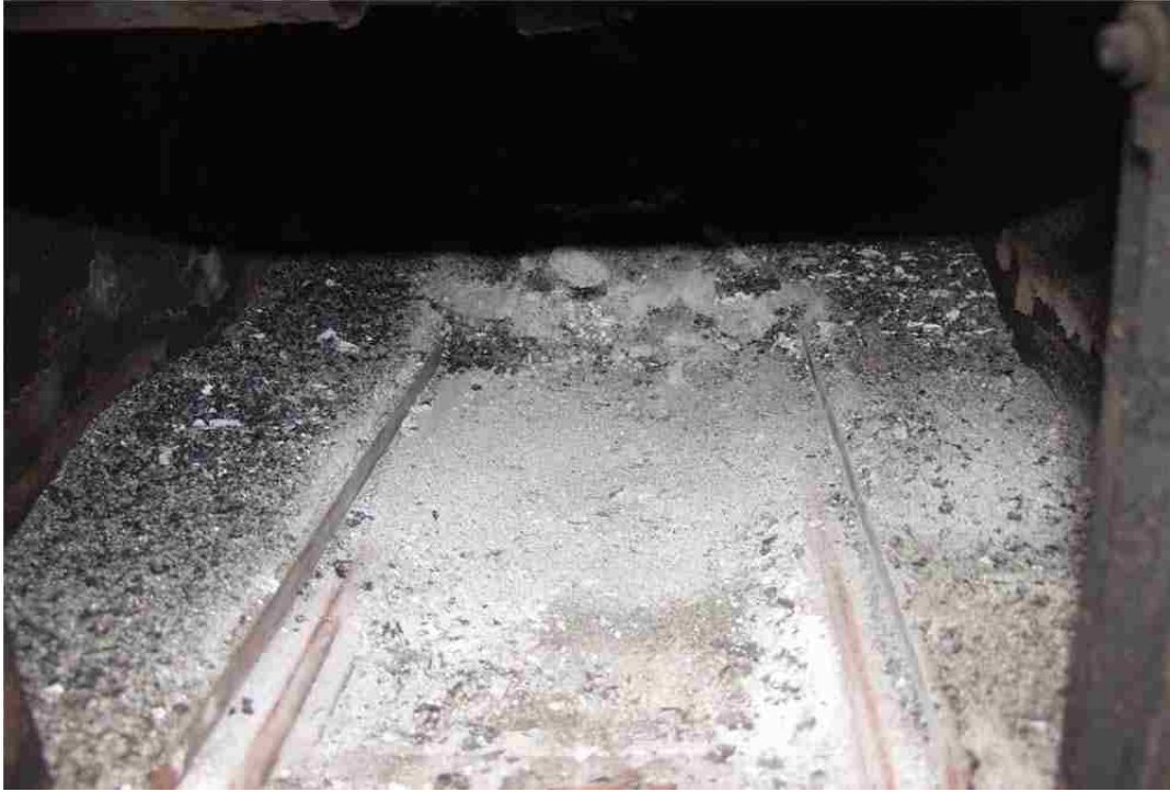
Figure 3.6. Firebox Ash Buildup.
