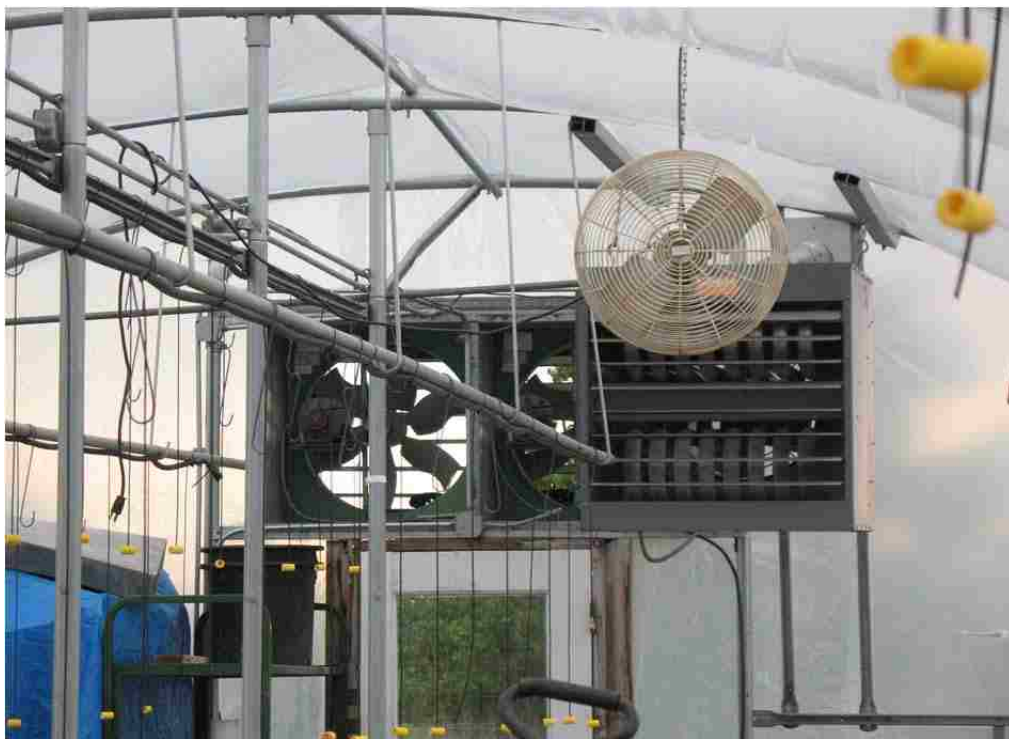
Figure 1.6. Overhead Modine Heating Unit. Windmaster Ventilation Fans are in the background.
