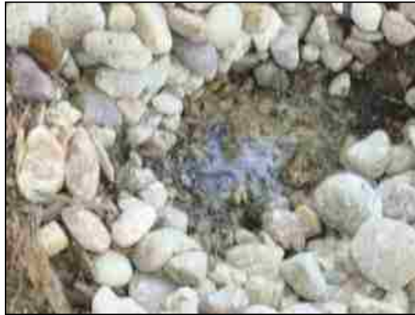
Rock-protected berm outlet (south side) showing overflow seepage.
