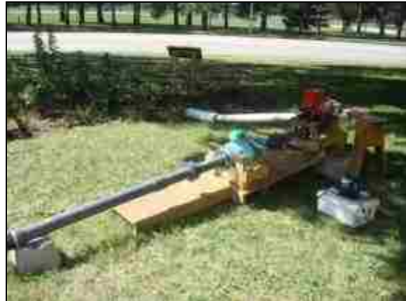
Flow meter/valve delivery system at inlet(9/23/10)
