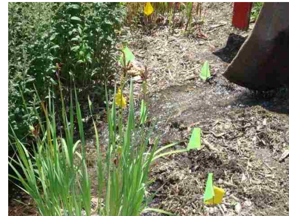
Figure 36. Influent from the simulator system is shown entering through the burlap sack (used for erosion control). Note the hydraulic flow path to outlet indicates poor retention.
