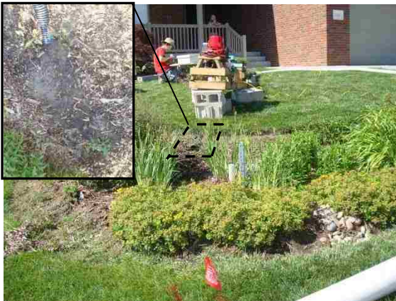
Figure 35. Rain garden connected to roof by buried black corrugated pipe emerging at the top slope of the cell. Insert photo shows closer look at inlet, which shows evidence of scour and sedimentation. Note the severe slope of the yard, which poses a challenge to residential rain garden performance.
