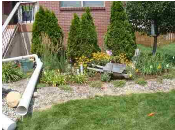
Figure 47. Inundated rain garden hugging foundation of home. Two roof downspouts contribute influent flow on either side of the garden.
