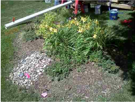
Figure 33. Rain garden installed on steep slope more than 30 ft. from downspout. Note heavily rock-armored overflow weir
