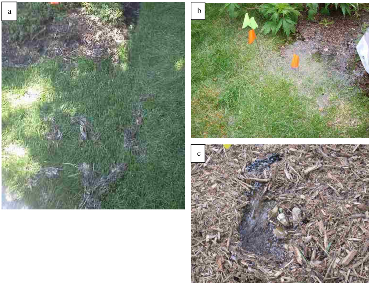
Figure 24. Photographs of failed overflow structures. (a) Outflow is at a low spot of the berm. (b) Lack of overflow structure. (c) Erosion of berm
