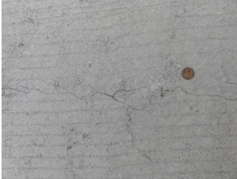
Figure C-4 Cracking in Dannon Way southbound conventional concrete deck at 1 year.
