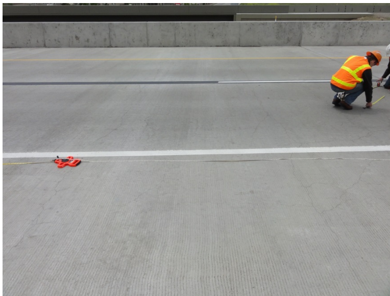
Figure C-1 Reflection cracking from half-deck concrete panels in 8200 South northbound conventional concrete deck at 1 year.
