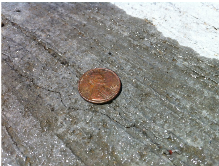
Figure 4-13 Cracking in Dannon Way southbound conventional concrete deck at 2 months.
