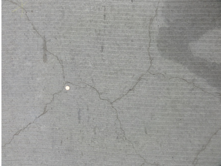
Figure C-2 Cracking in 8200 South northbound conventional concrete deck at 1 year.
