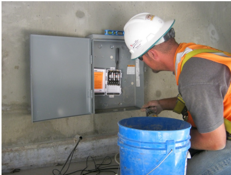
Figure 3-8 Data logger mounted in box.
