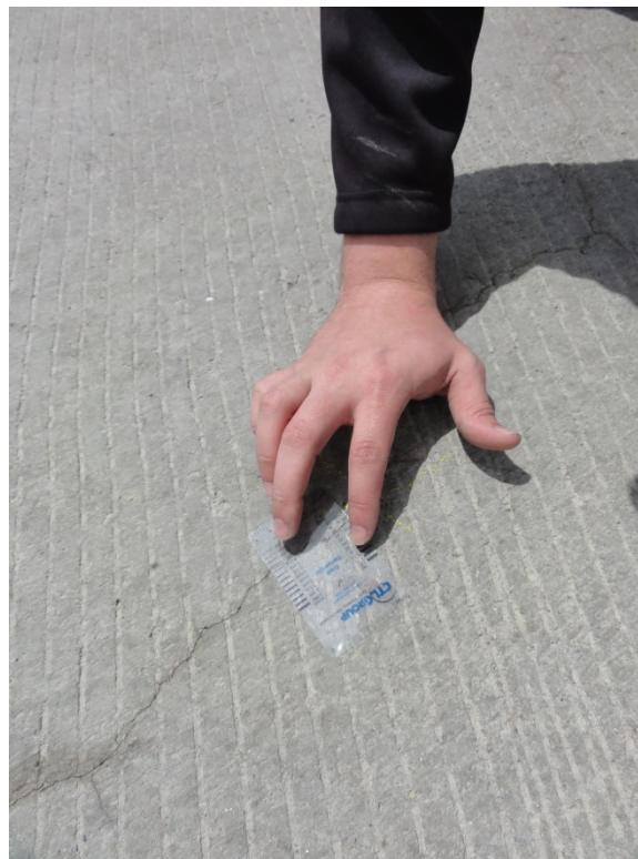
Figure 4-15 Cracking in 8200 South northbound conventional concrete deck at 1 year.
