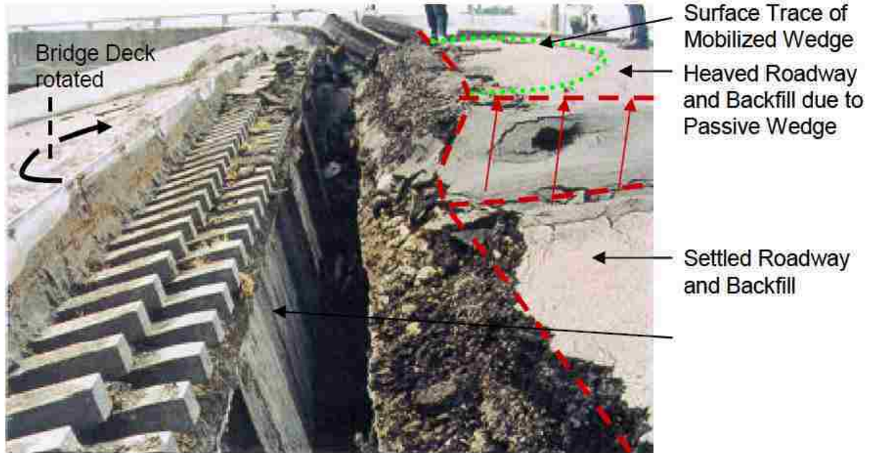
Figure 2.12. Asymmetric backfill heave pattern at Wushi highway bridge abutment in Taiwan, adapted from Shamsabadi et al. (2006).
