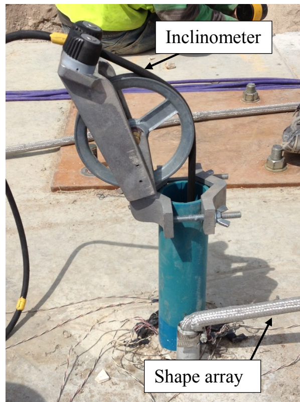
Figure 3.35. Inclinometer and shape array at the top of the pile cap.
