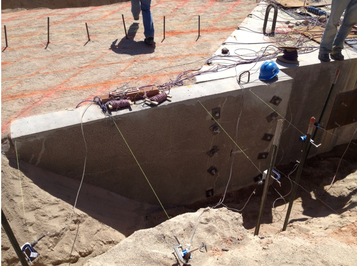
Figure 3.42. Wingwall string potentiometer instrumentation.
