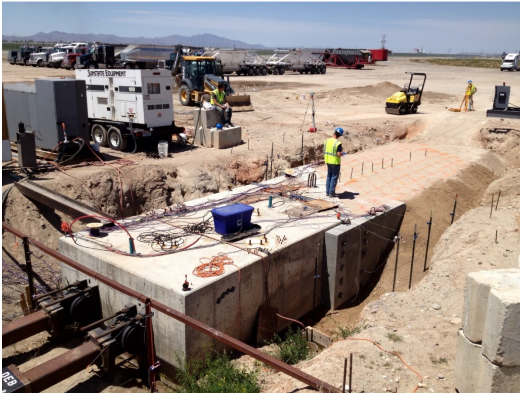
Figure 3.19. Densely compacted sand backfill with a 2H:1V slope at the edges for 45° skewed abutment.
