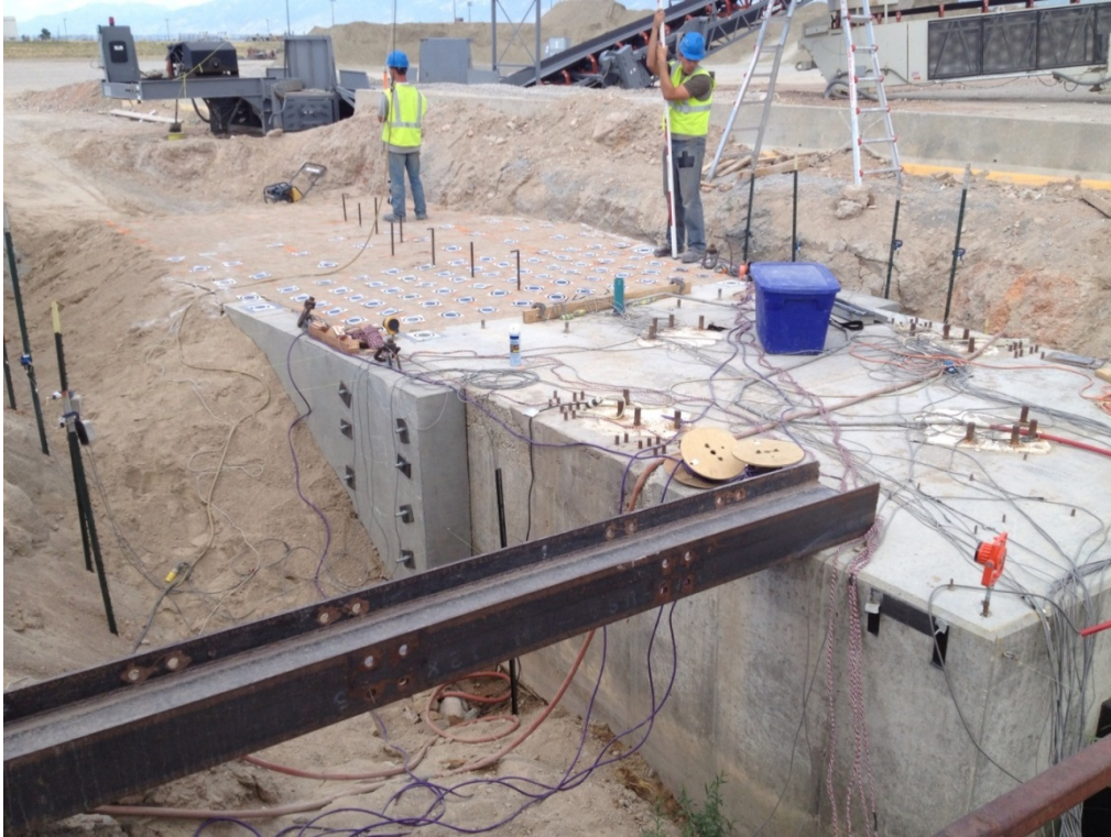
Figure 3.20. Densely compacted sand backfill with a 2H:1V slope at the edges for non-skewed abutment.
