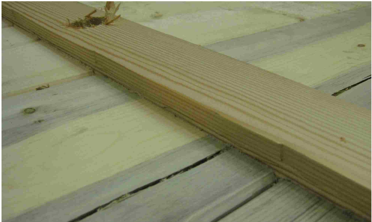
Figure B-2: Dovetail Member Crushing (Wall 1).
