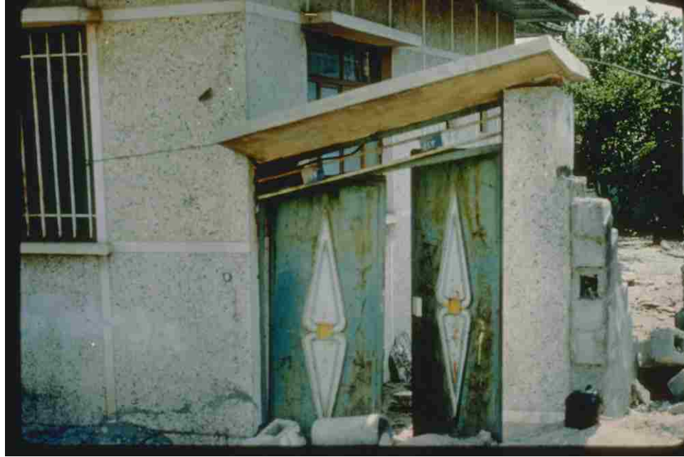
Figure 2-8: Differential settlement in Iran 1990 after NOAA/NGDC - M. Mehrain, Dames and Moore.
