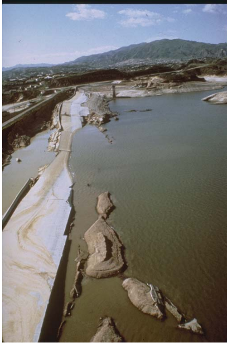
Figure 2-10: Flow failure at lower San Fernando Dam 1971 after NOAA/NGDC - E.V. Leyendecker, U.S. Geological Survey.
