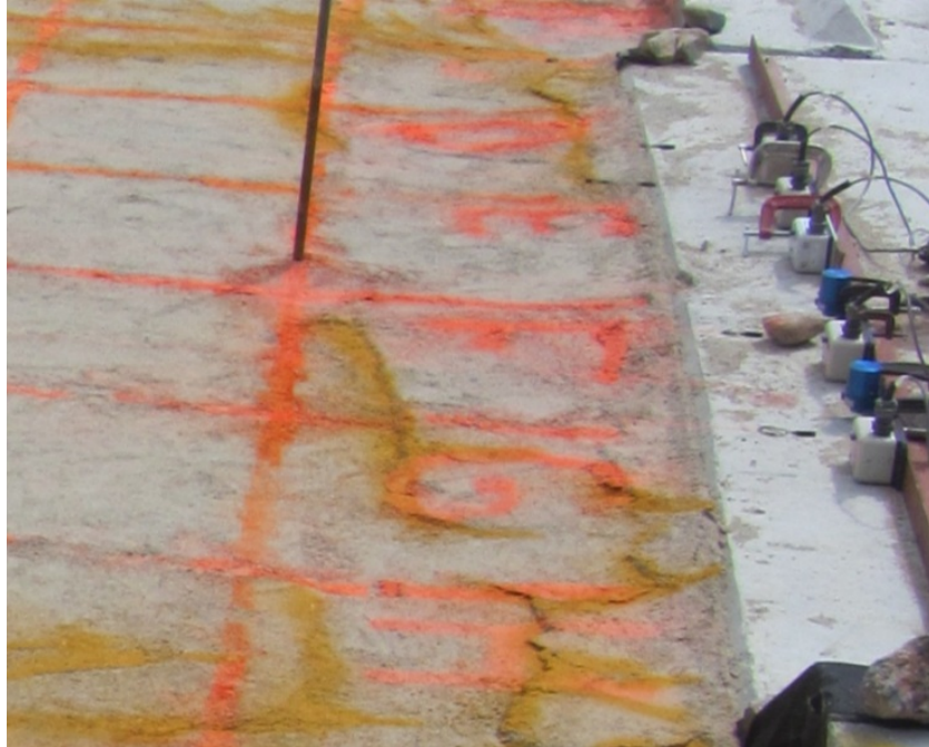
Figure 7-10: Transverse compression cracks at test completion
