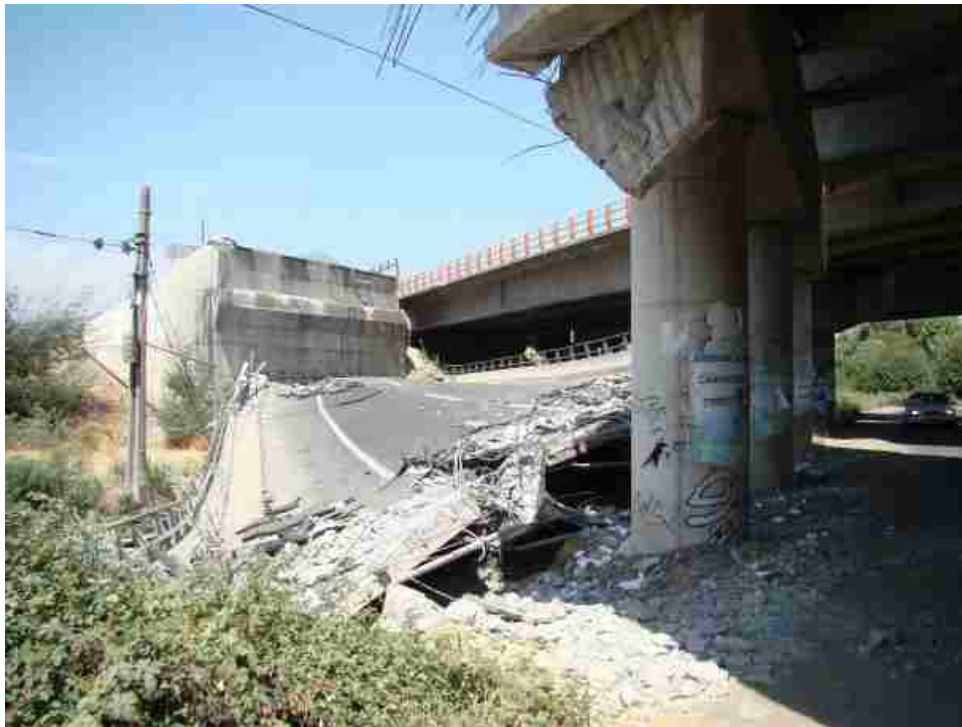
Figure 2-22: Collapse of skewed bridge deck adjacent to a functioning normal bridge. Chile Maule earthquake, 2010 (Unjohn, 2012)
