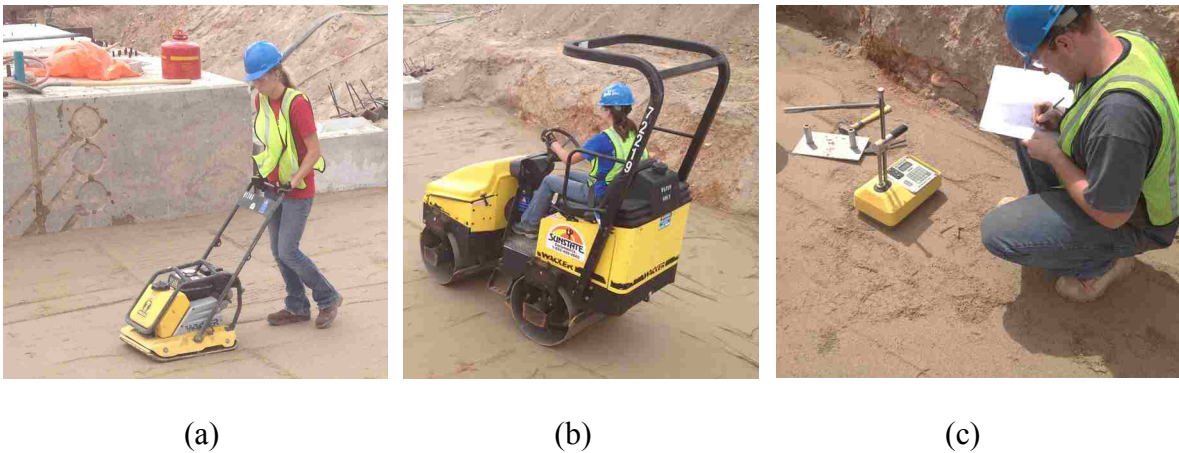
Figure 3-33 Backfill compaction including (a) vibratory plate compaction, (b) vibratory roller compaction, and (c) nuclear density gauge evaluation.
