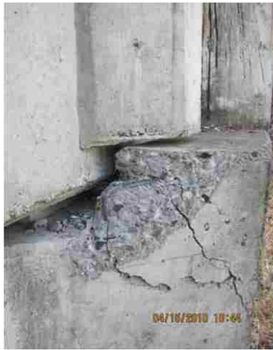
Figure 2-21: Damaged shear key at abutment. Chile Maule earthquake, 2010 (Elnashai et al., 2010)
