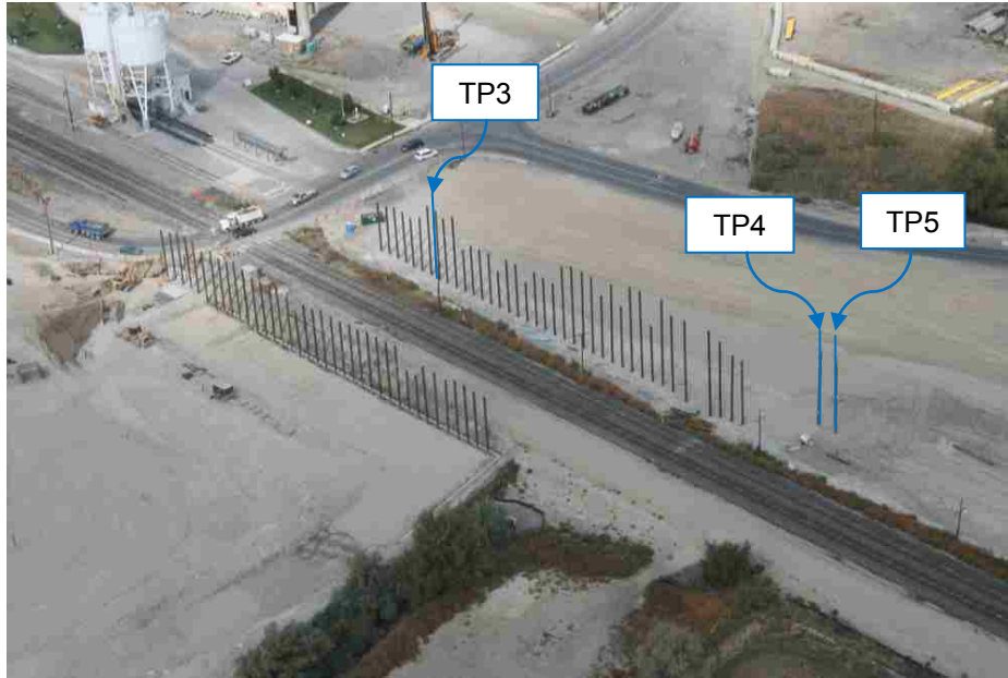
Figure 3.7: Piles for the Pioneer Crossing bridge over UPRR prior to wall construction.
