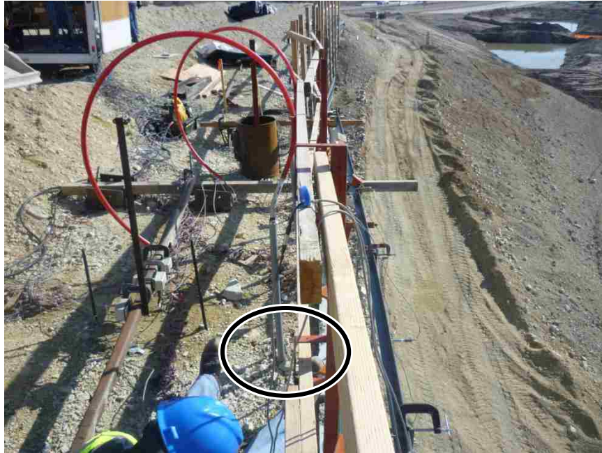
Figure 5.31: Shape Array casing in line with TP4 separated from wall by a couple inches.
