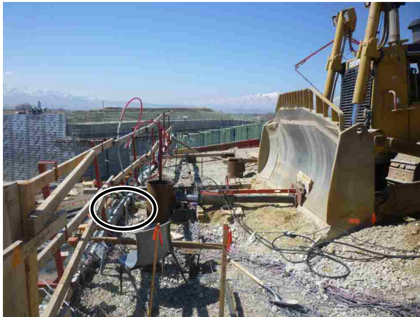
Figure 5.32: Shape Array casing in line with TP5 separated from wall by a couple inches.
