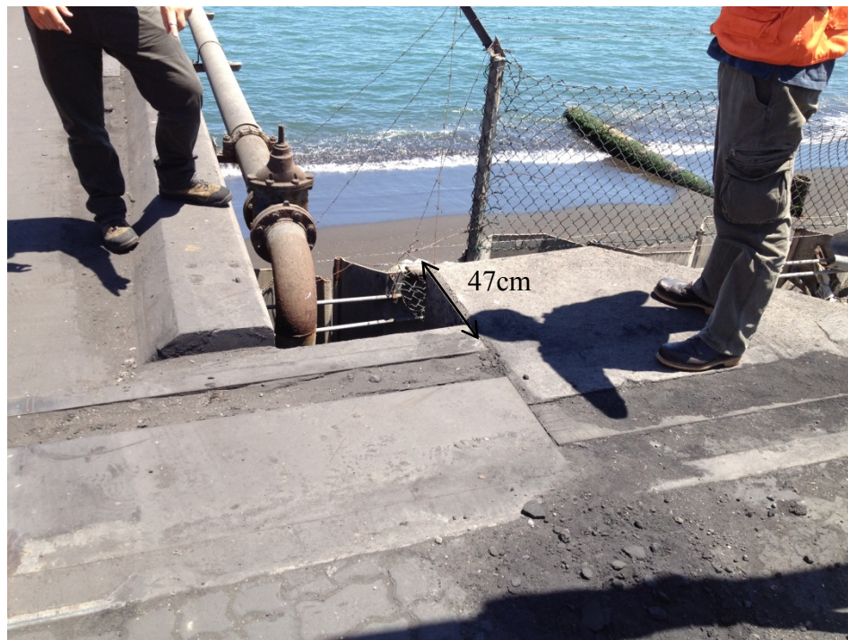
Figure 5-12: Displacement of Ground Relative to the South Coronel Pier
