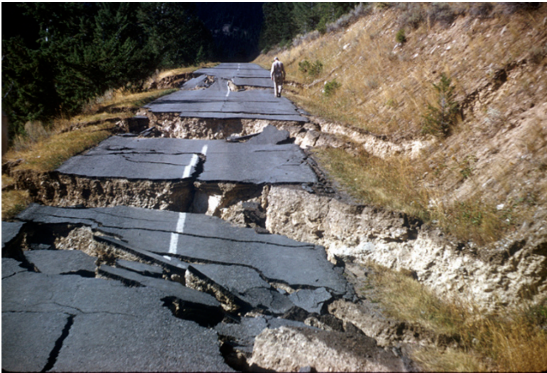
Figure 1-2: Road Damaged by Lateral Spreading, Photo by R. B. Colton (Idaho Geological Survey n.d.)
