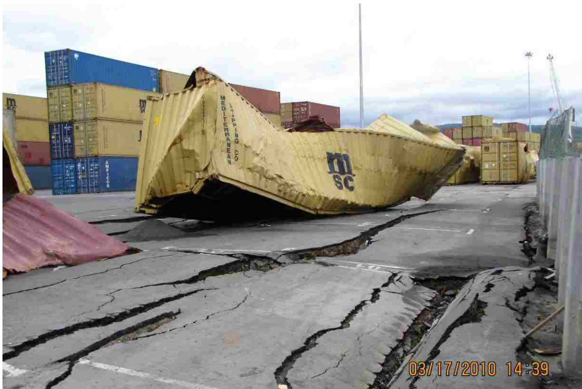
Figure 5-17: Toppled Containers at the Port of Coronel (GEER 2010)
