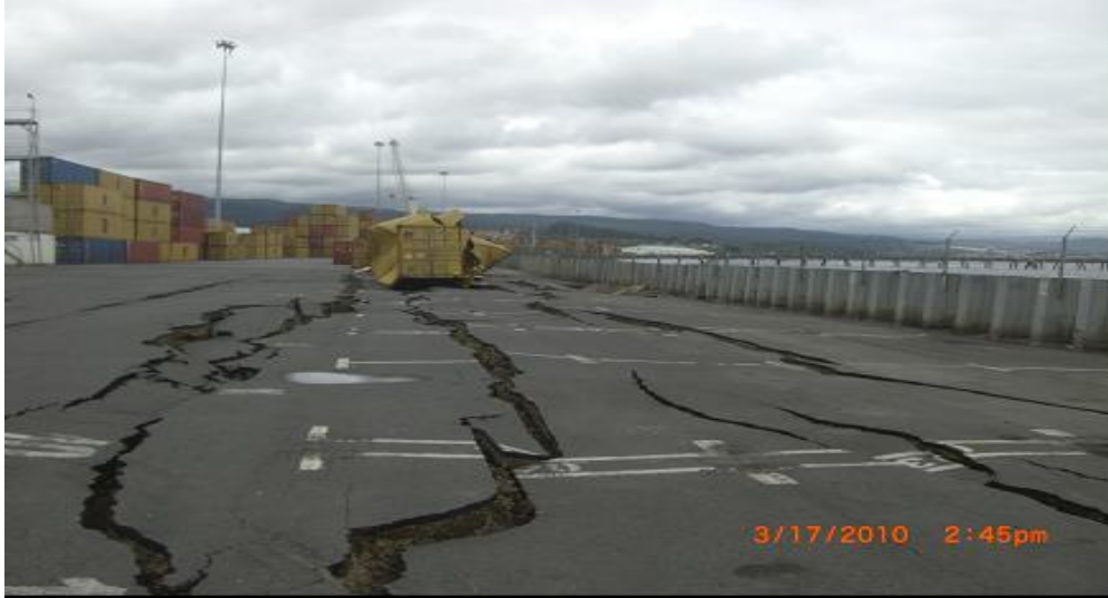
Figure 5-3: Lateral Spreading Cracked the Asphalt Between the Coronel Piers (GEER 2010)
