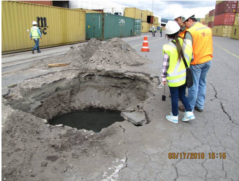
Figure 5-18: Sink Holes at the Port of Coronel (GEER 2010)
