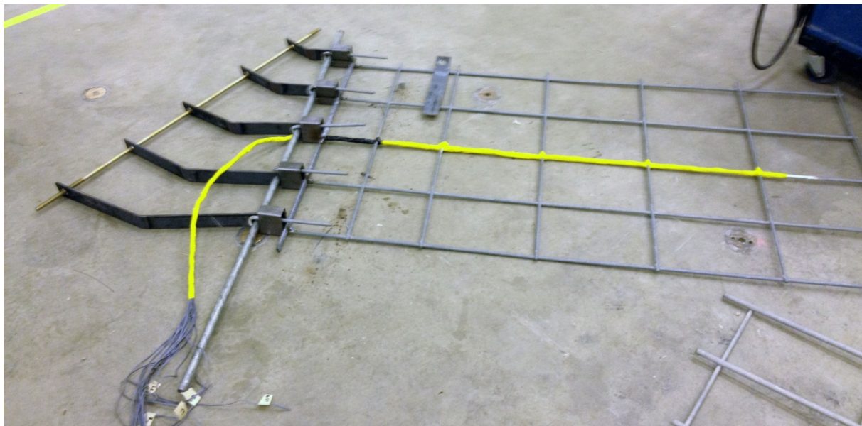
Figure 3.19: Angled Adapter Connectors attached to Reinforcement Grids to Accommodate the Skewed Shape
