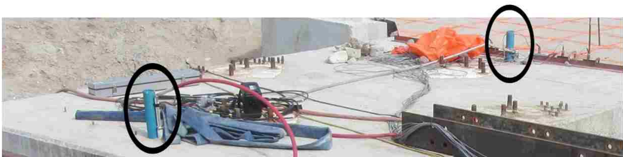
Figure 3.26: Inclinometer locations on top of pile cap
