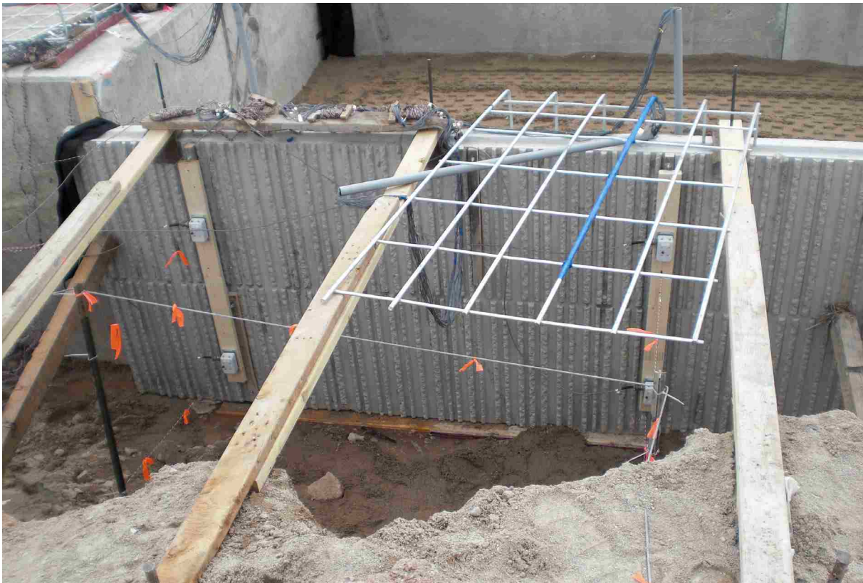
Figure 4-15: String pots to measure wall deflection.
