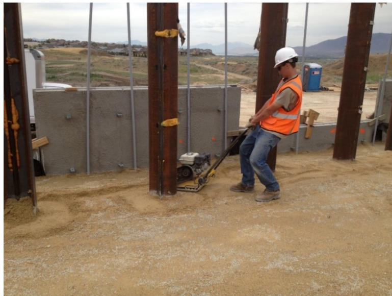
Figure 3-5: Plate Compaction Between MSE Wall and Piles Adjacent to The MSE Wall
