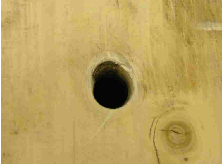
Figure 4-3: Elongation of Hole at the Bottom of Wall in In-Plane Lateral Load Test
