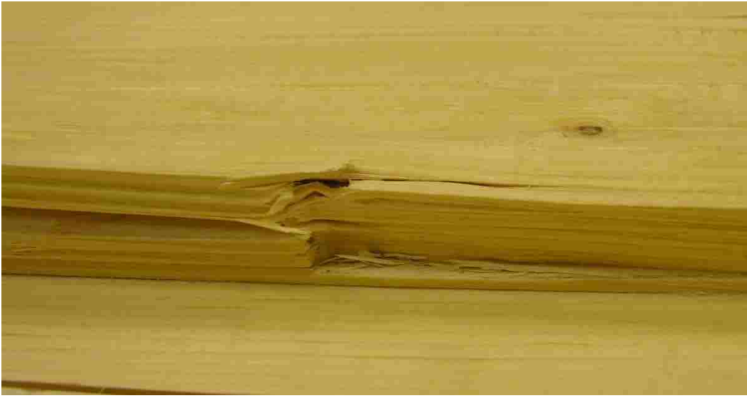
Figure A-5:Crushing of Dovetail Section in Racking Wall
