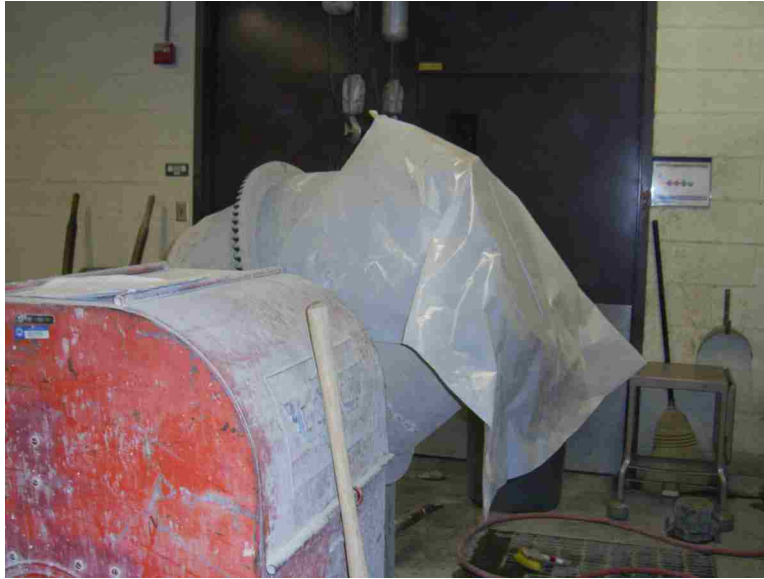
Figure 3-3: Concrete mixer opening covered with plastic sheeting.
