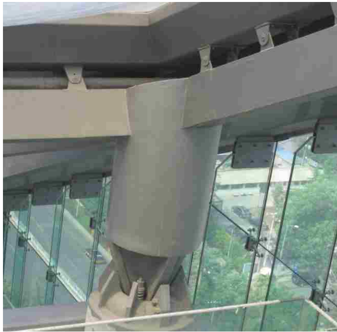
Figure 39: Close Up of Ball and Socket Joint
