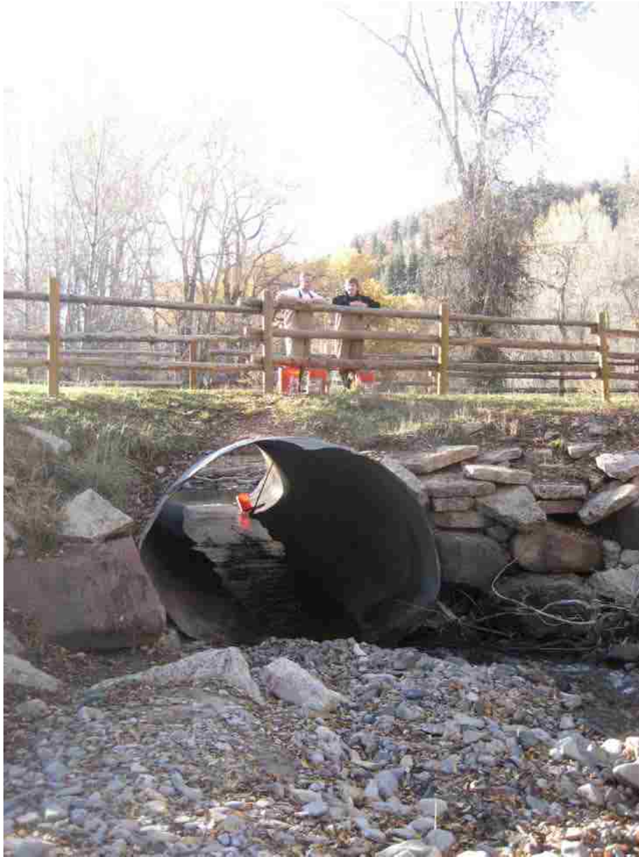
Figure 4-2: Deposition at the Salt Creek Culvert Entrance.
