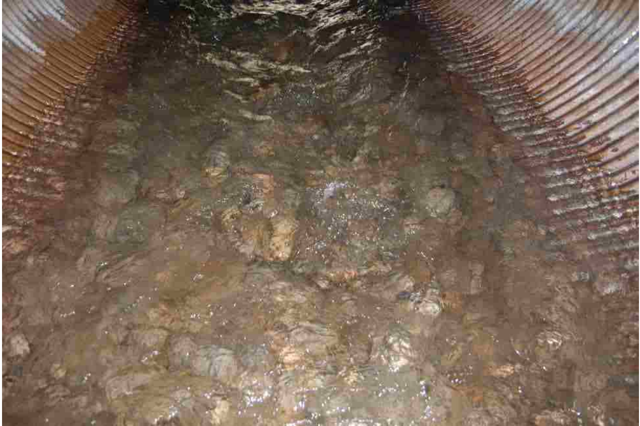
Figure 4-13: Sediments Deposited in the Salt Creek Culvert Barrel.
