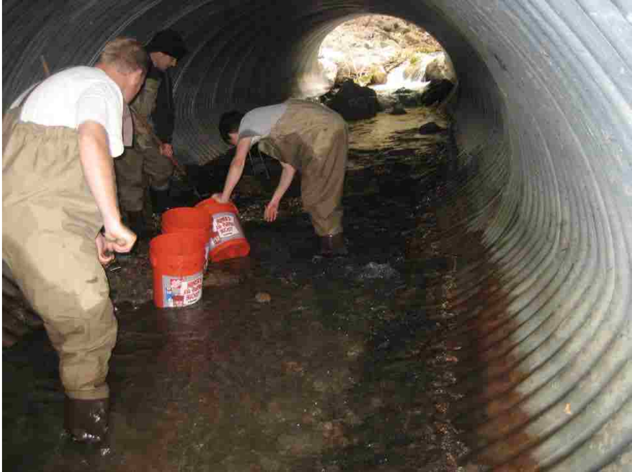
Figure 3-14: Ed Kern, Dan Jones, and Evan Cope Work to Remove Sediments from the Summit Creek Culvert Barrel.
