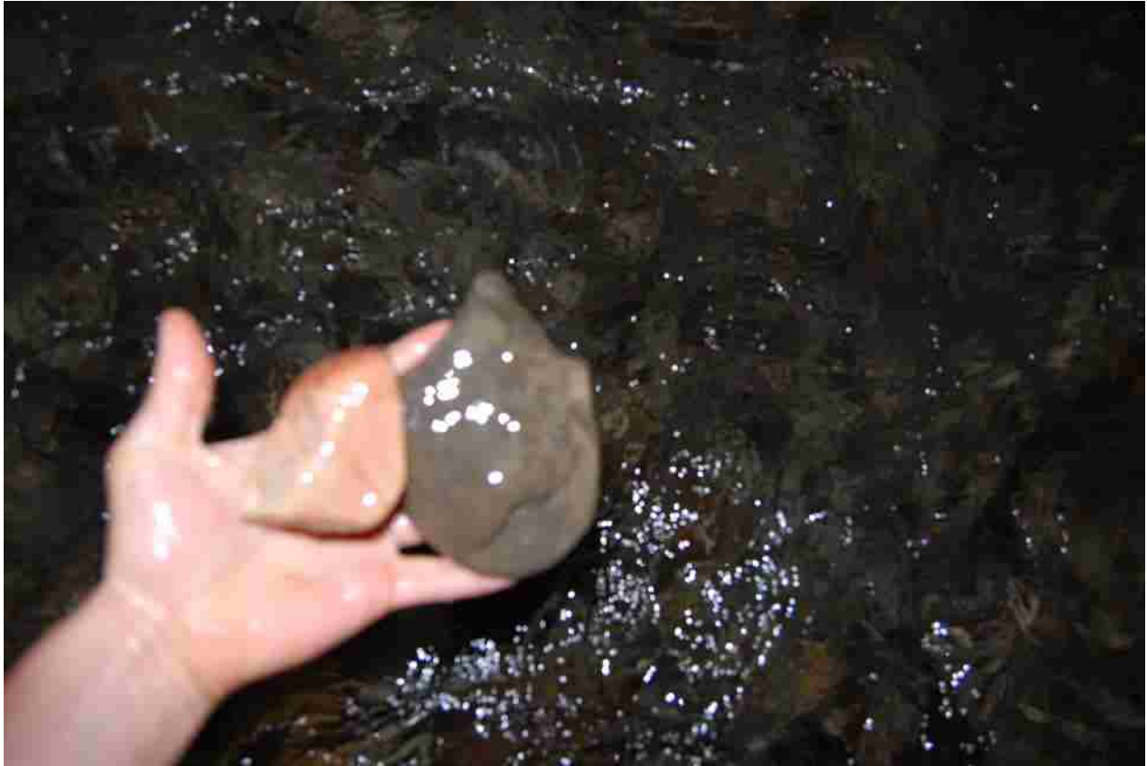
Figure 4-12: Sediment Deposits Found in Salt Creek Culvert Following High Flows.
