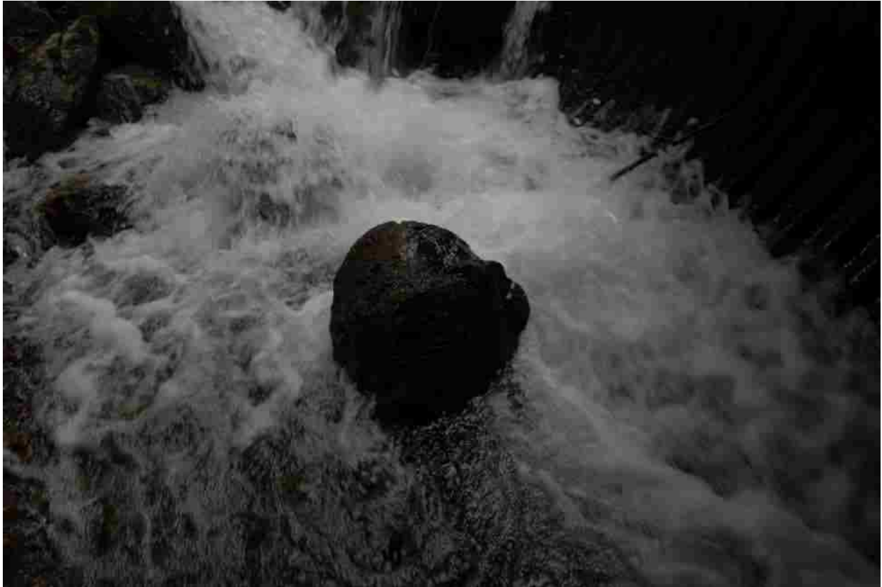
Figure 4-14: Small Boulder Settled inside the Summit Creek Culvert.
