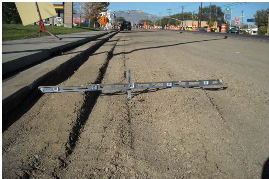
Figure 3-13: Significant rutting occurring hours after emulsion-treated base construction.
