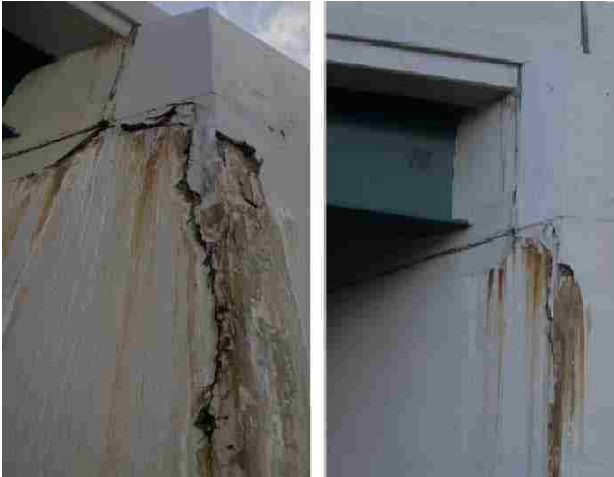
Figure 2-17: Cracking, Distress Observed at Ohio Skew Bridge Wingwall (Steinberg & Sargand, 2010)
