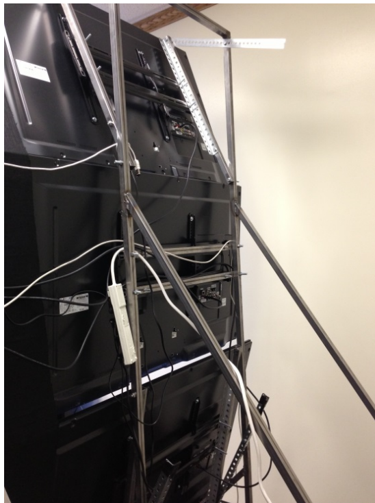
Figure 2-7: Three monitors attached to a steel frame with adjustable tilting arms and Rocketfish wall mounts.
