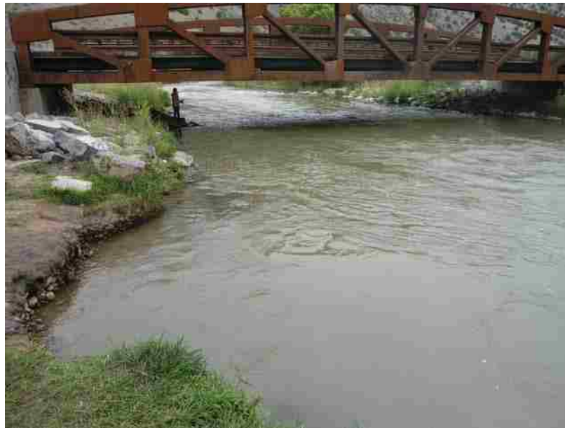
Figure 2-4: Abrupt Change from Riprap to Streambank, Causing Downstream Scour. Flow from Top to Bottom (picture taken by Evan Cope).
