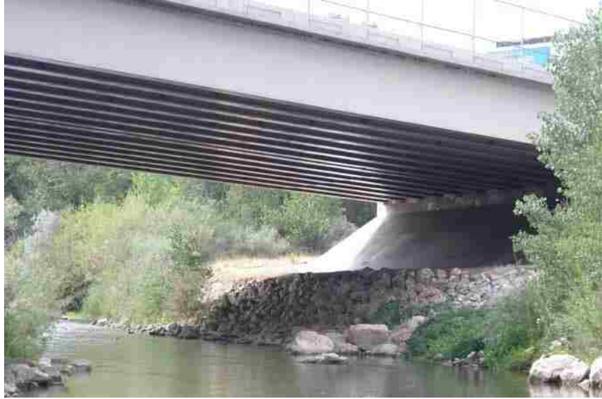
Figure 2-3: Riprap Used to Protect a Bridge Abutment. Flow From Top to Bottom (Picture Taken by Evan Cope).
