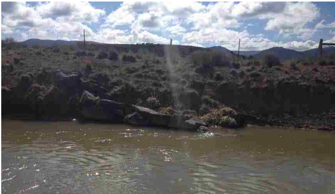
Figure 3-9: Steep Vane Slope has Increased Steambank Erosion. Flow from Right to Left. (Picture Taken by Evan Cope)
