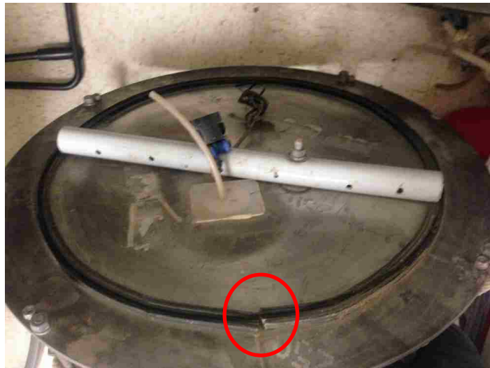
Figure 20: Gap Marked with Red Circle Indicating Gap in O-Ring
