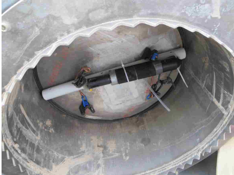
Figure 16: Probes Zip Tied to the Top of Chamber Lid
