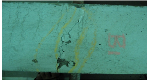
Figure 14 Crack in SFRC.
