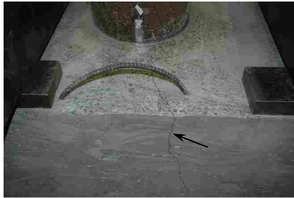
Figure 4-2: Initial Cracking in Specimen 1 (East-West)
