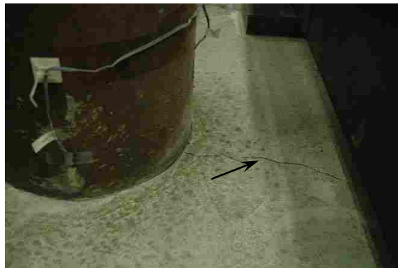
Figure 4-10: Initial Cracking of Specimen 3 (East-West)
