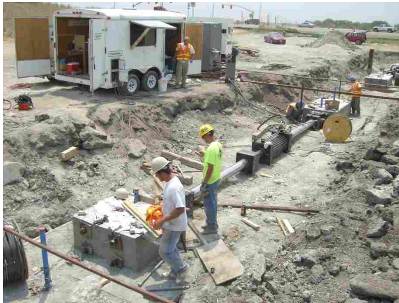
Figure 4-10 Photo of actuator setup between caps 1 & 2.
