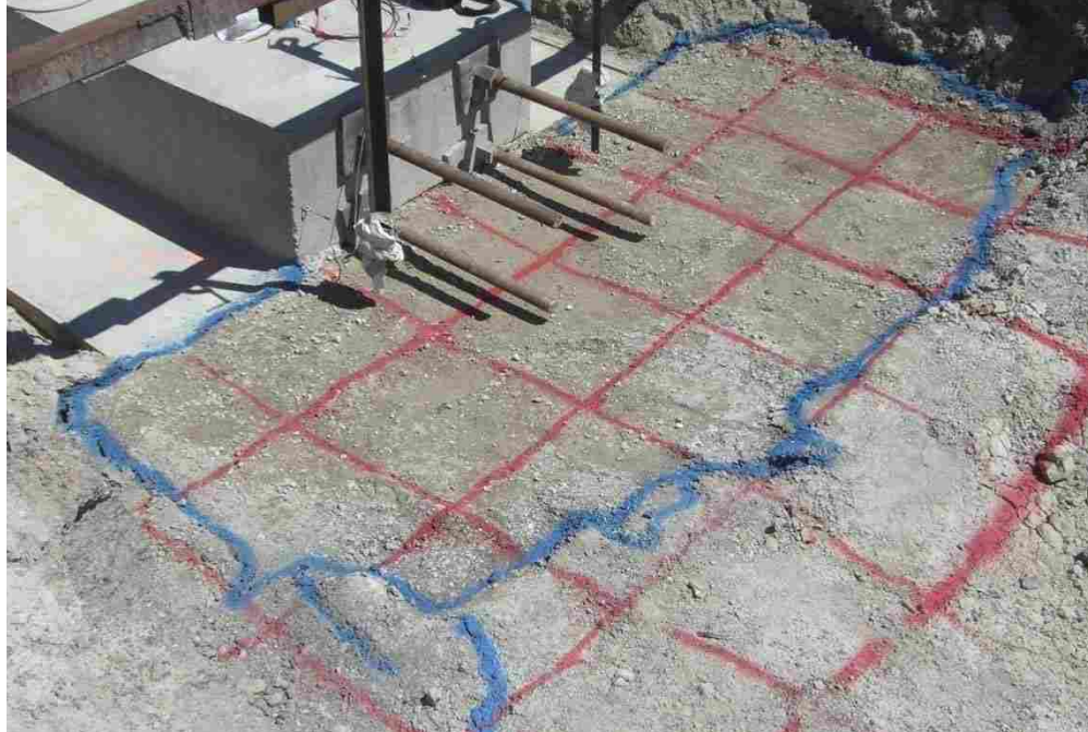
Figure 6-9 Photograph showing the flowable fill surface failure condition and that the zone acted as a rigid soil block.
