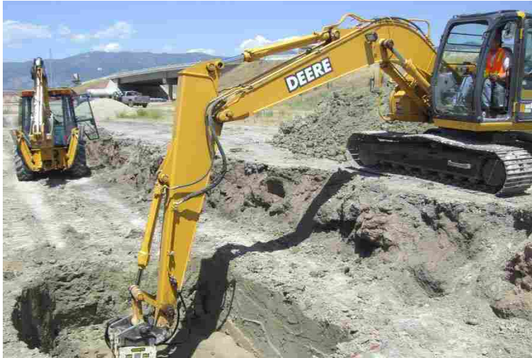
Figure 5-1 Compaction of fill under future pile cap 4 using a hydraulic plate compactor attached to the arm of a track hoe
