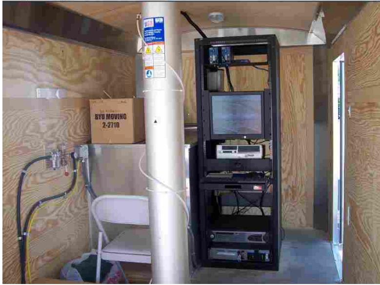
Figure 3-8: The inside of the data collection trailer
