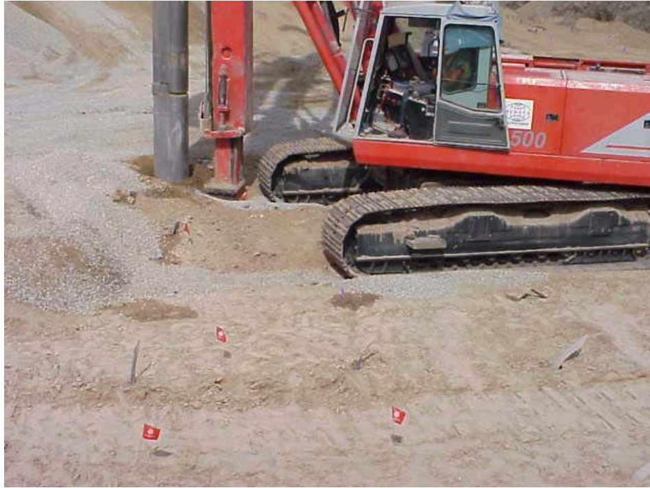
Figure 8-5 Photo of water draining from the wick drains during installation of a stone column.
