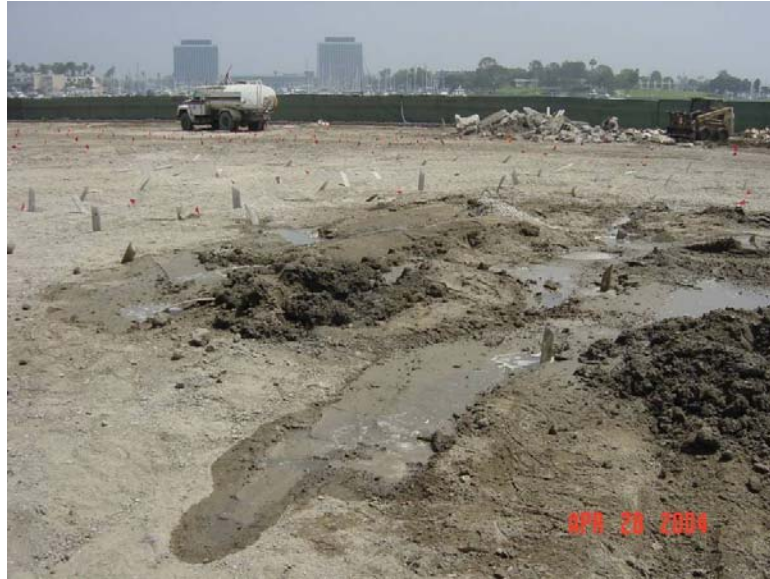
Figure 2-7 Water escaping through previously installed wick drains during stone column installation (source, Hayward Baker, Inc.).
