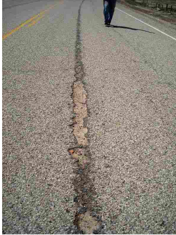
Figure 4.3 Pothole along chip seal joint.
