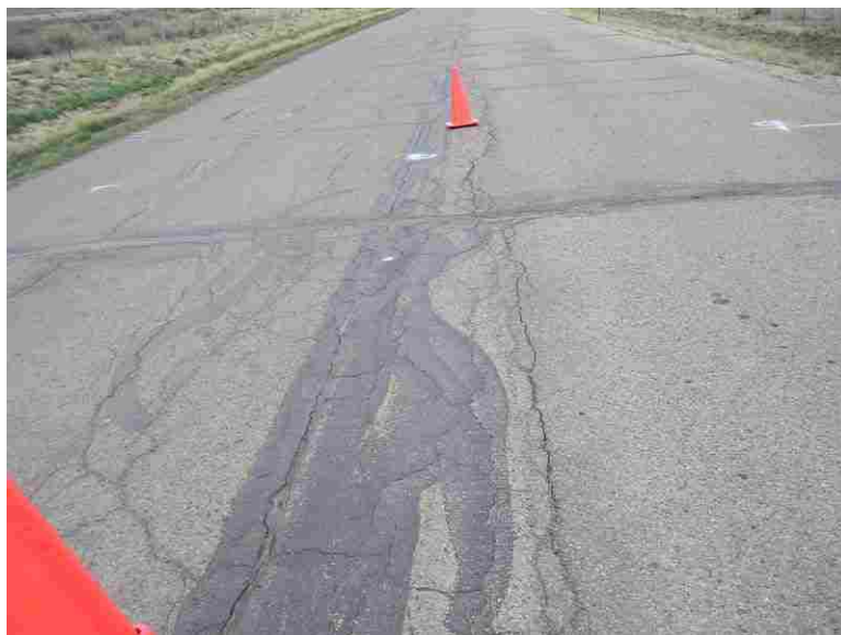
Figure 3.1 Existing pavement distress.
