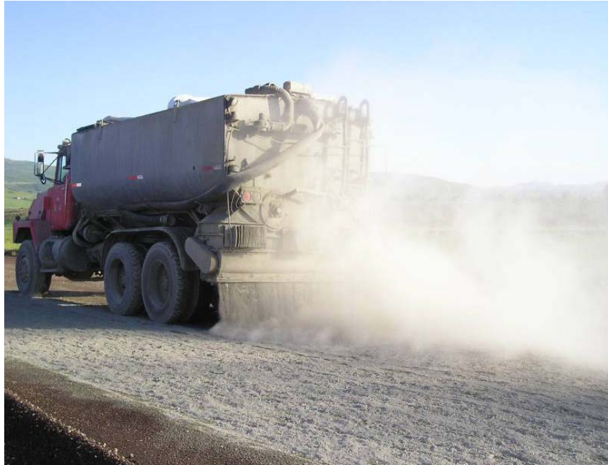
Figure 2.3 Fugitive cement dust associated with applying dry cement using a pneumatic spreader.
