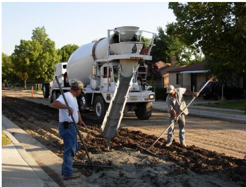
Figure 2.6 Application of cement slurry in an FDR project directly from the chute of a ready-mix truck.
