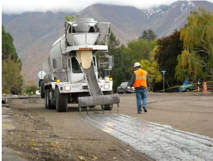
Figure 2.5 Application of cement slurry in an FDR project using a slurry spreader.
