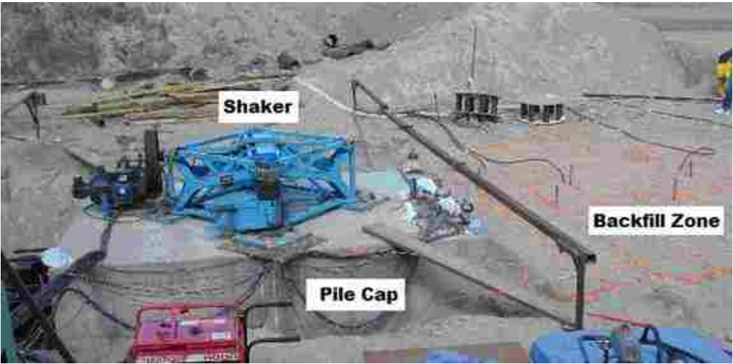
Figure 3.5 Photos of test site and equipment setup
