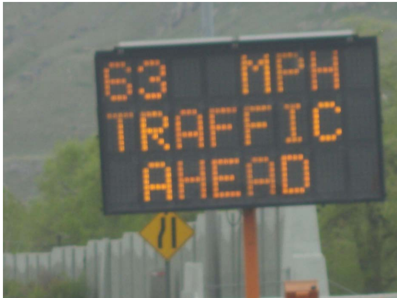
Figure 3-9 First message displayed on VMS 2 (taken by Aaron Wilson).
