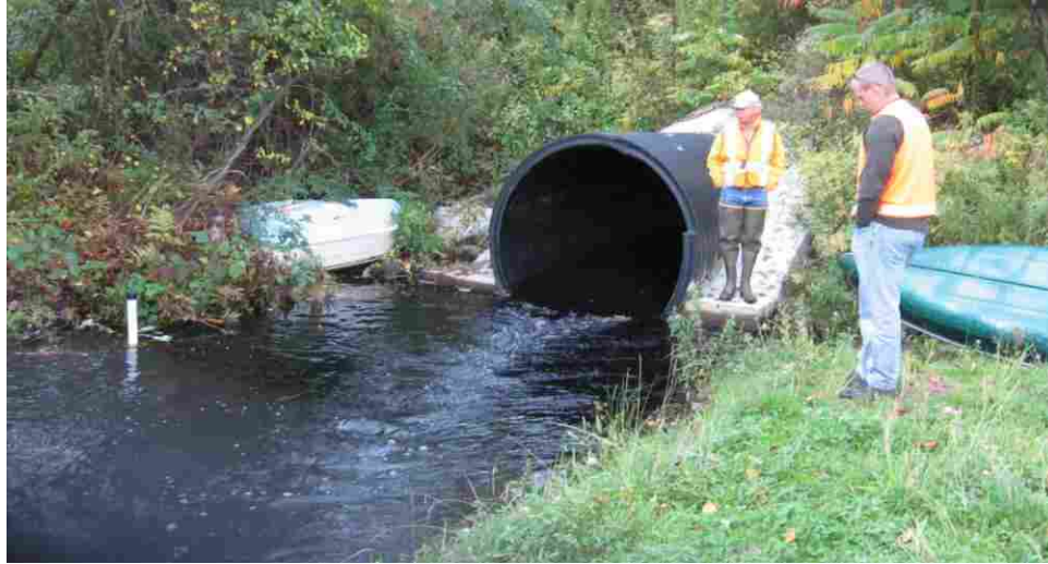
Figure 3-7: Culvert retrofit on Alewife Creek near Cape Elizabeth, Maine. Tailwater weir is submerged.
