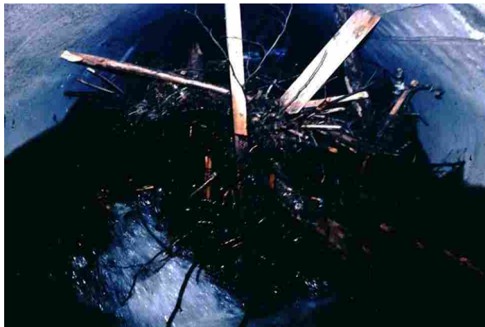
Figure 3-3: Debris caught on a baffle. (CALTRANS 2007)
