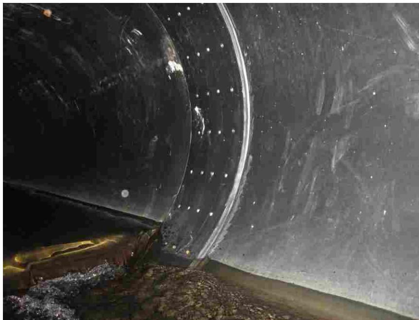
Figure 3-9: Welding of culvert segments. Attachment used as opportunity to provide anchoring for baffle.
