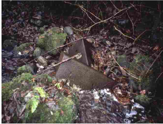
Figure 3-2: Failure due to insufficient anchoring. (CALTRANS 2007)
