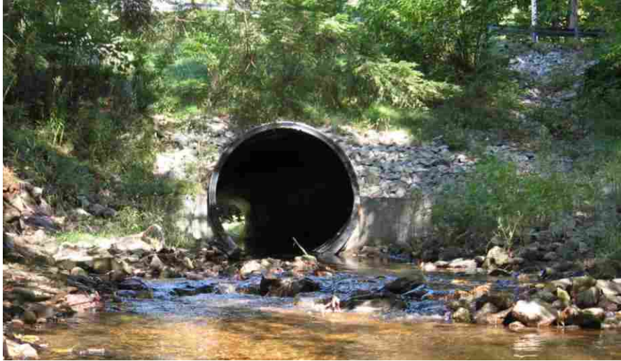
Figure 3-14: Outlet of Falmouth, Maine slip lined culvert retrofit. Rock tailwater grade control also shown.
