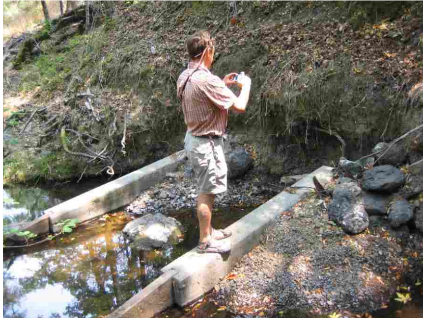
Figure 3-5: Erosion flanking tailwater control weirs at John Hatt Creek.
