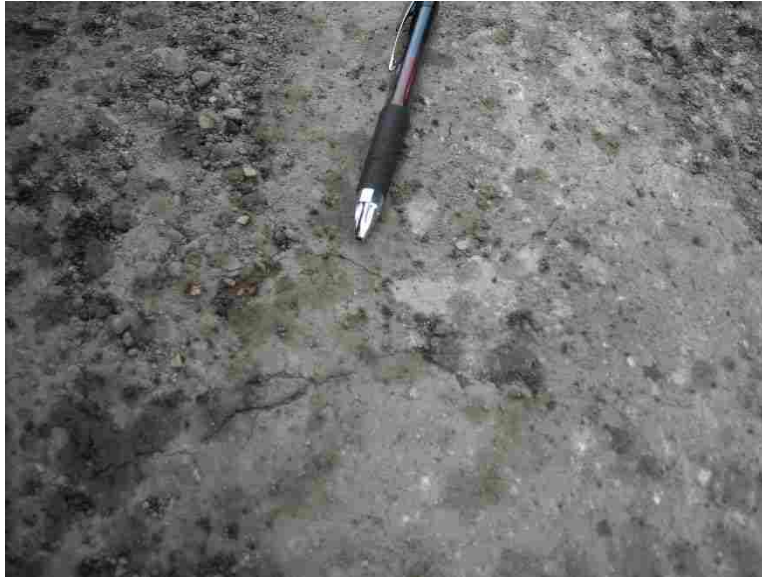
Figure 4-24: Fine cracks in CTB surface after microcracking.
