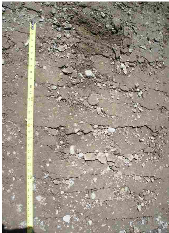
Figure 4-23: CTB surface damage due to slow vibratory roller speed during microcracking.
