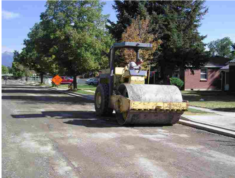
Figure 2-4: Microcracking using a vibratory roller.
