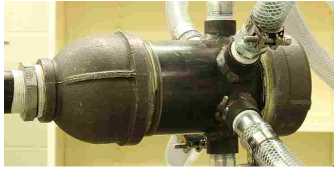
Figure 3.9: Flow dividing plenum. The plenum was made from 4 inch pipe.
