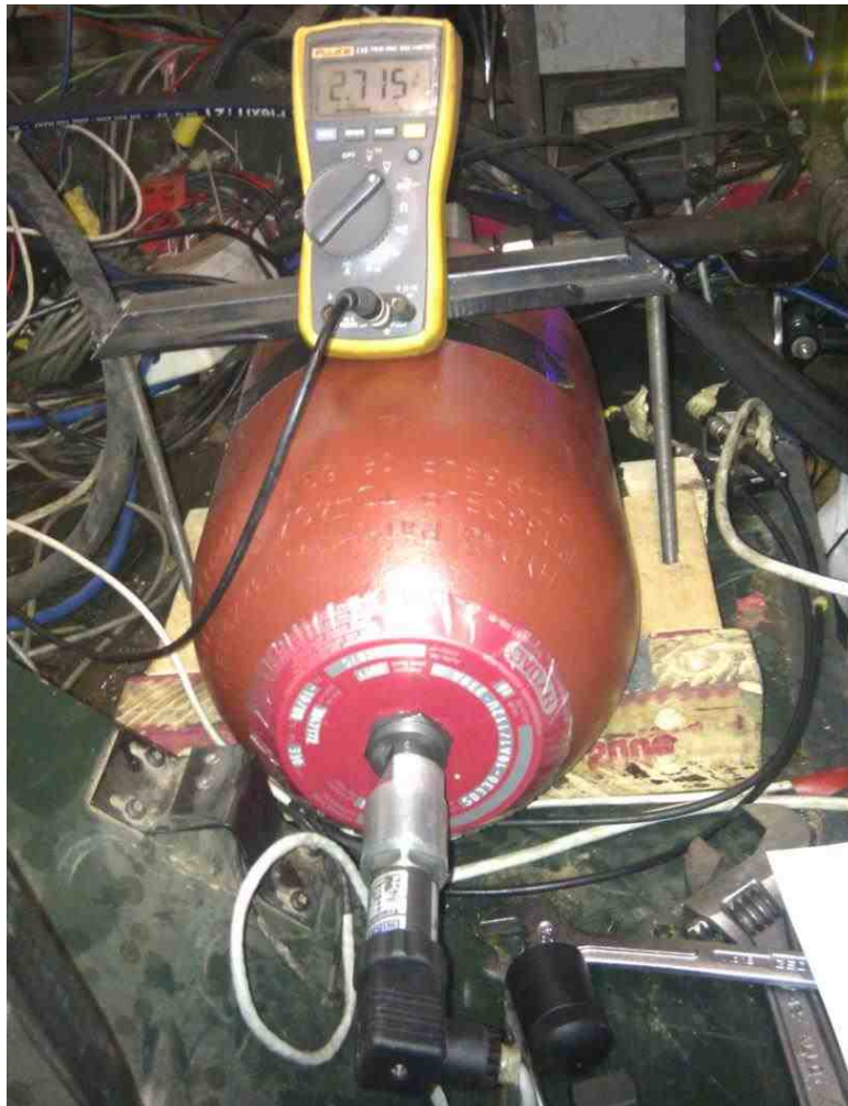
Figure 75 10 ℓ bladder type accumulator being charged to 7 MPa
