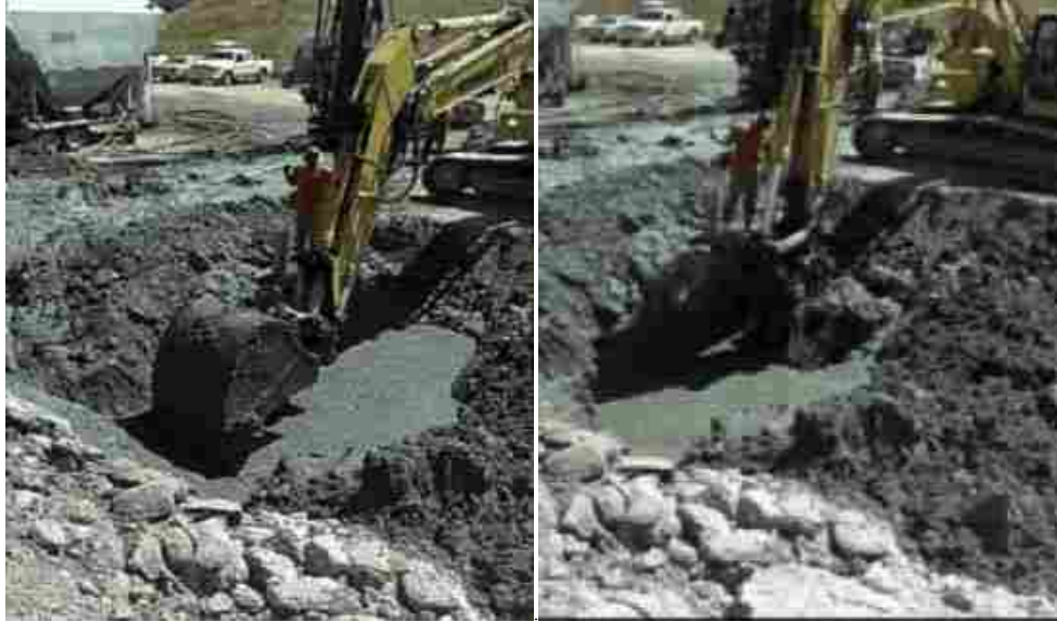
Figure 4-12 – The process of mixing the insitu soil with the jet grout spoils.
