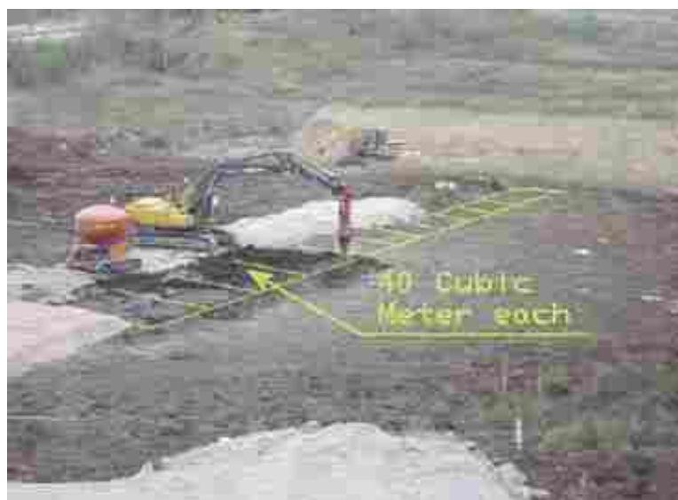
Figure 2-7 - Schematic illustration and photograph of mass stabilization by blocks method (ALLU website 2007).
